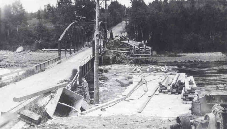
Construction of the Stevens Bridge over the Reversing Falls, South Blue Hill 1926
