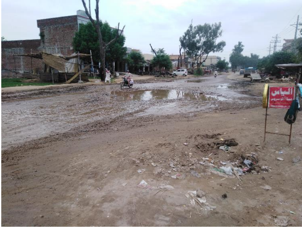
Figure 11: incomplete Portion of road during site visit
