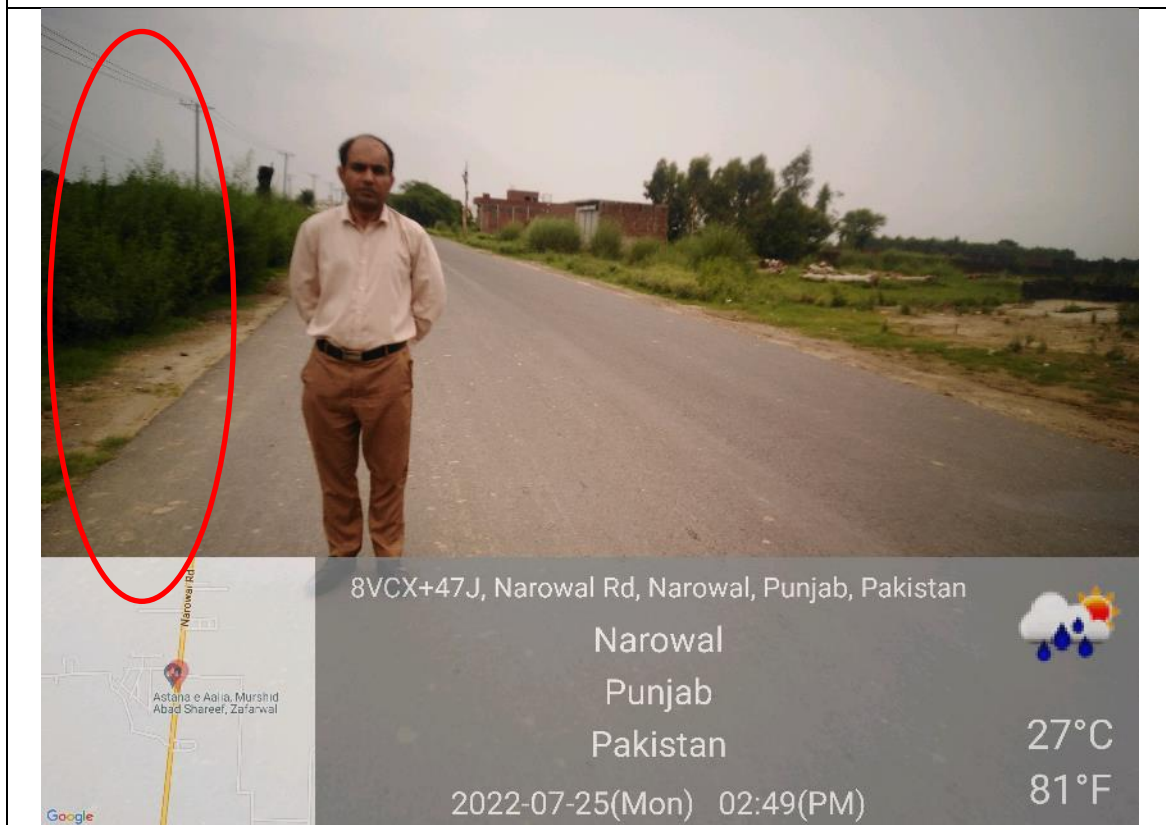
Figure 4: A view of constructed single way road without maintenance of shoulders
