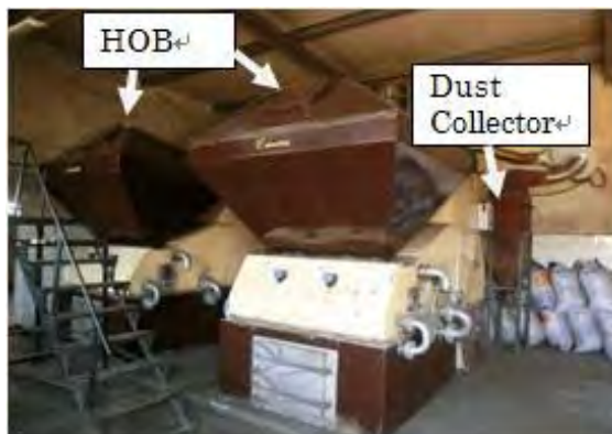
Fig. 4-13 Main HOB and Dust Collector
