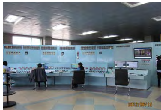
Fig. 4-10 Operation Monitoring Control Panel for Boiler #1 to #4
