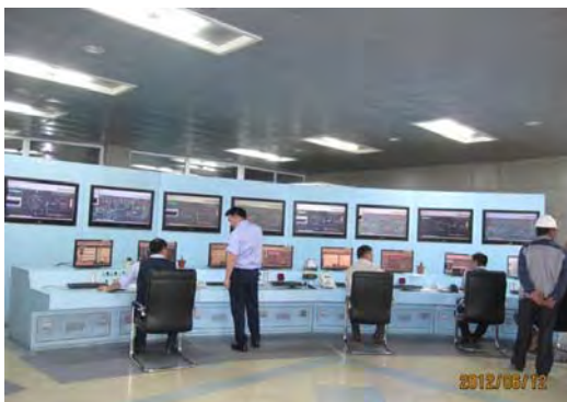
Fig. 4-9 Operation Monitoring Panel for Turbine #1 to #3
