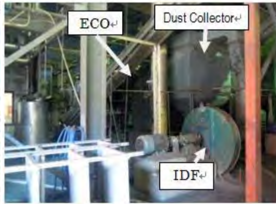
Fig. 4-16 Rear View of Industrial Boiler
