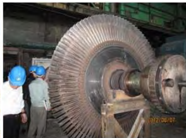
#5 turbine rotor in overhaul inspection Updated in 1995, overhaul inspection in 2007
