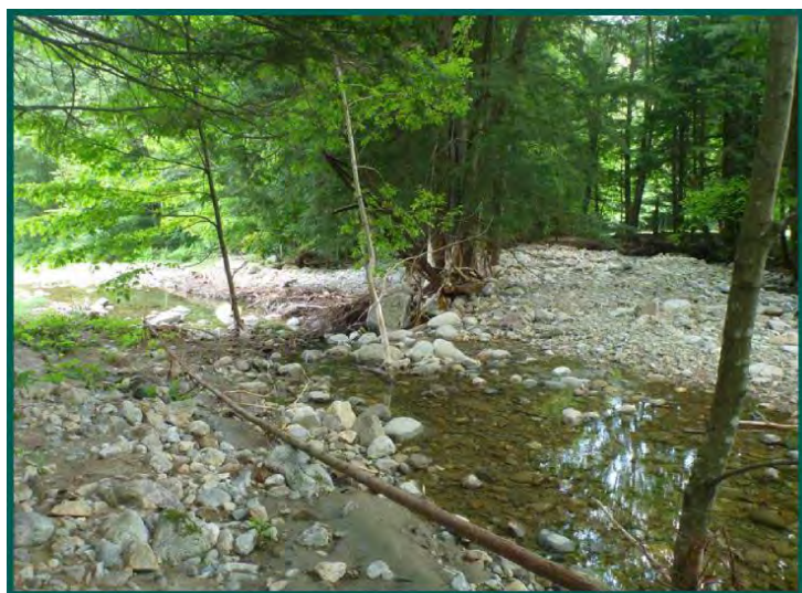
Merriam Brook in Surry on July 31, 2013. The original channel (to the right) filled in with rock transported from upstream, forcing the channel to break through the bank, cutting a new channel for itself at the southern end of the homeowner's lawn (to the left). (Source- NHDES)
