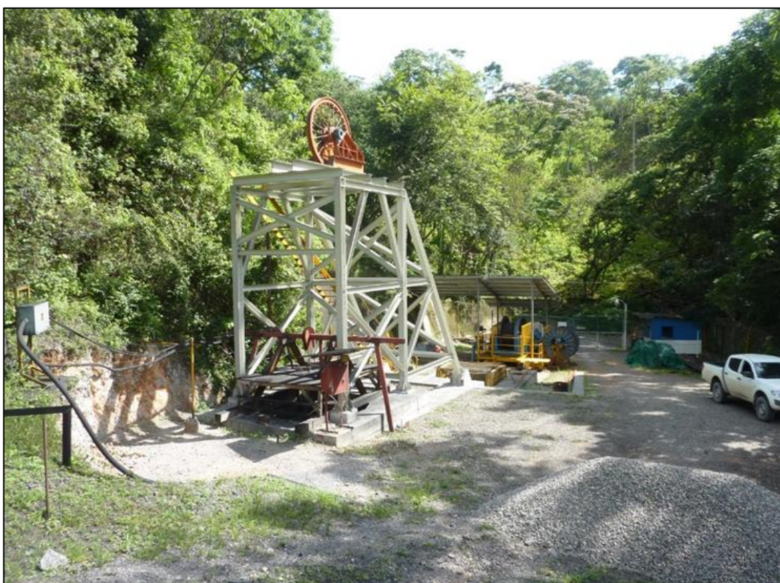
– Shaft headframe installed over 2.7 m borehole - Bonanza raise bore hole (shaft) to 1100L (Figure 16.13)
