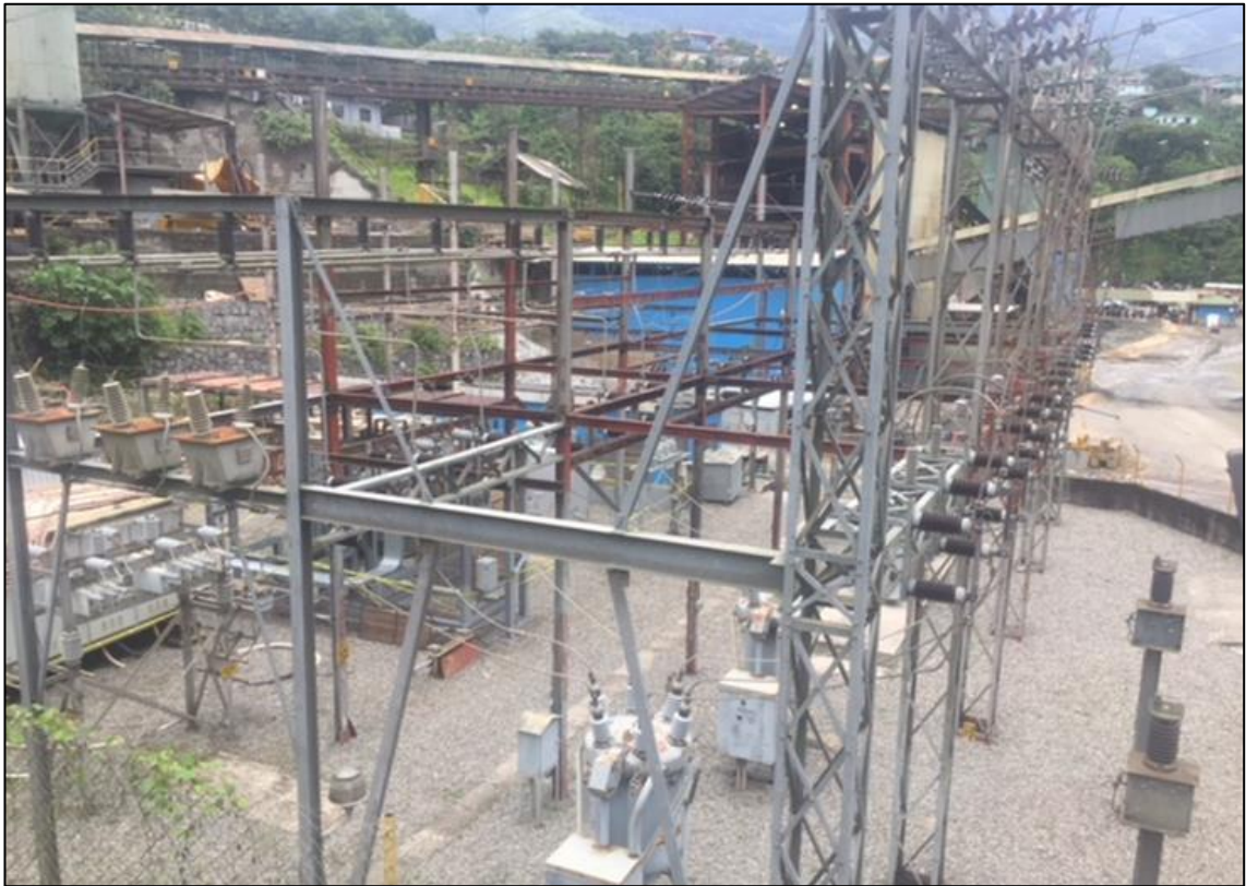
Figure 18.5 – 34.5 kV old substations
