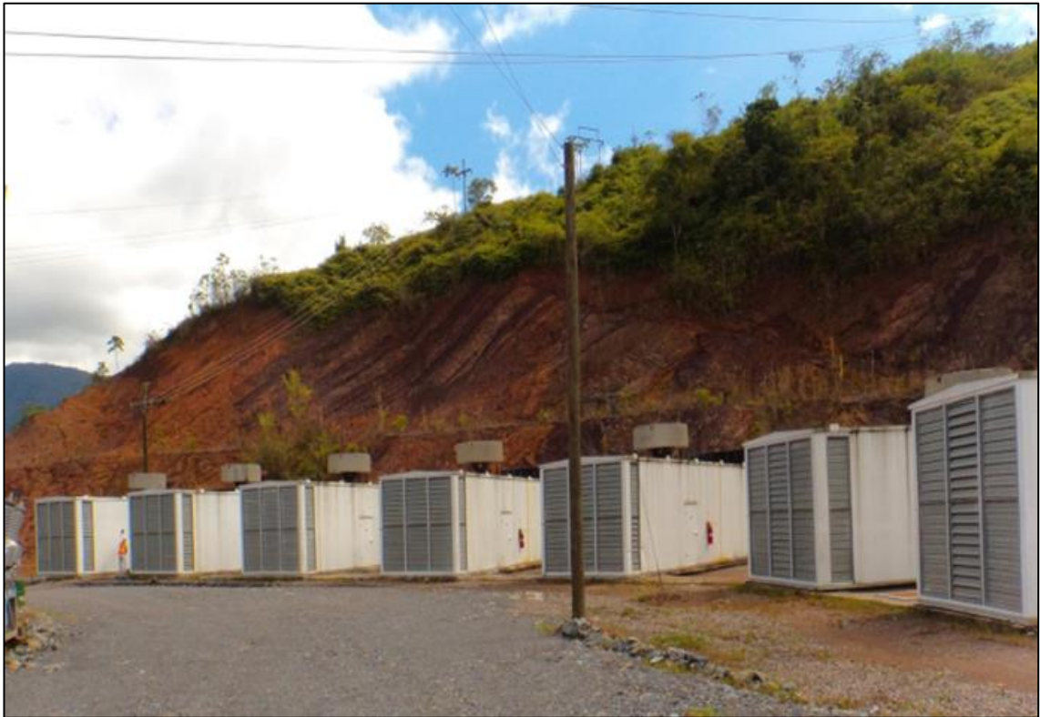
Figure 18.6 – CAT diesel generators
