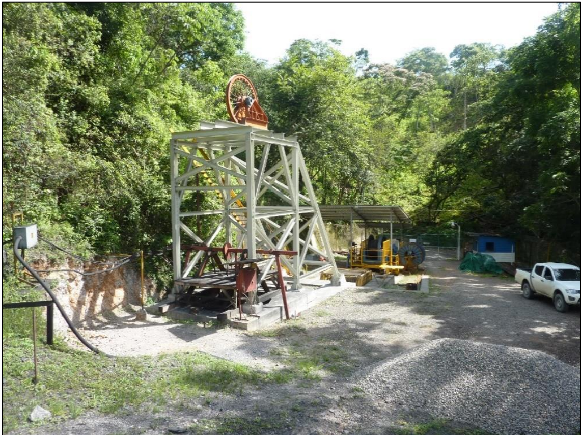
Figure 16.13 – Shaft headframe installed over 2.7 m borehole - Bonanza raise bore hole (shaft) to 1100L
