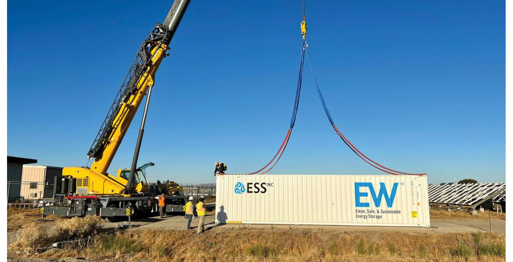
ESS flow batteries enable a steady supply of electricity from intermittent energy sources, such as wind and solar. They store up to 12 hours of energy and discharge it when needed. They can be built in shipping containers, like the one being installed in the picture here, or larger installations can be housed in a building. Credit: ESS Inc.
