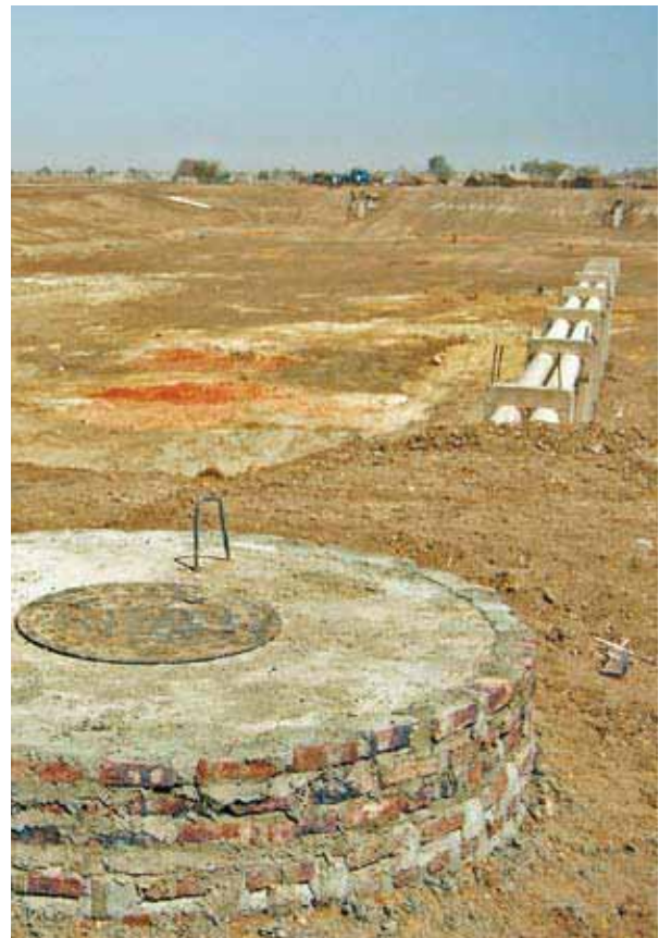
Settlement pond under construction at the Kenana Sugar Company, located near Kosti, which has recently invested heavily in the construction of water treatment facilities
