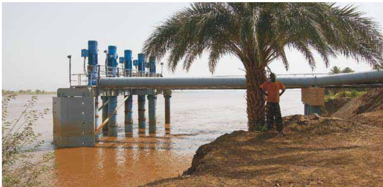
Riverbank erosion removed the supports of this irrigation pump intake system within months of its installation, and threatens to destroy it completely. Without mitigatory measures, the site is not suitable for such a project
