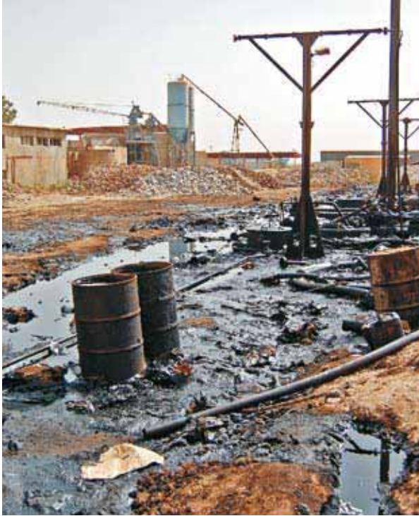
Fuel oil spillage at the Rabak cement factory, in White Nile state
