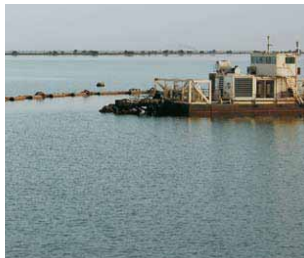
At the Roseires dam reservoir, a dredger is continuously used to remove sediment from the electric turbine water inlets. Soil washed from the Ethiopian highlands is the main source of the sediment
