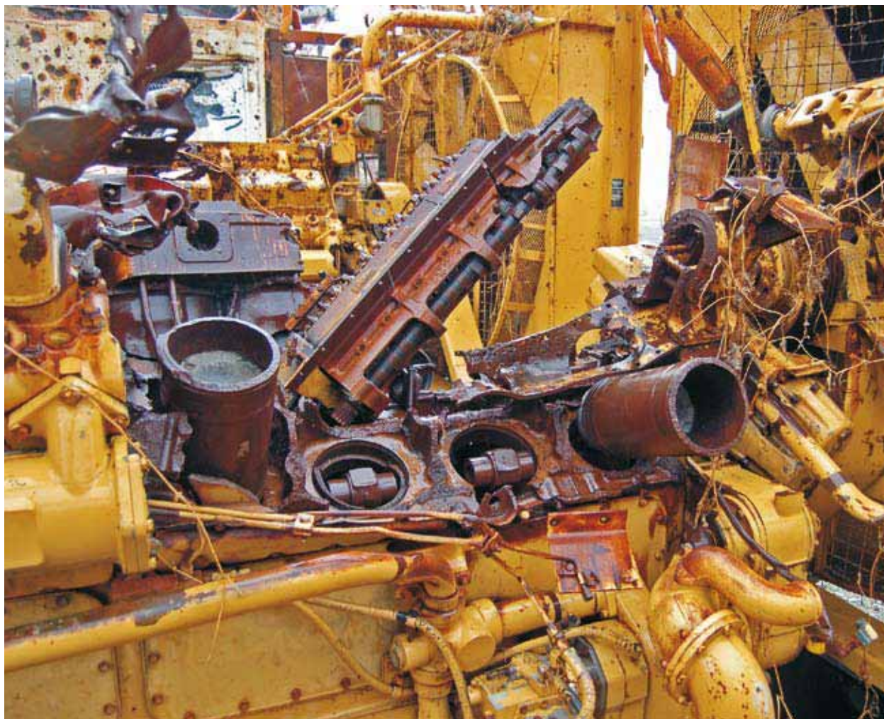
In 1983, southern military forces sabotaged these generators powering the Jonglei canal excavator. Plans to restart the giant water project constitute a major potential flashpoint for renewed conflict
