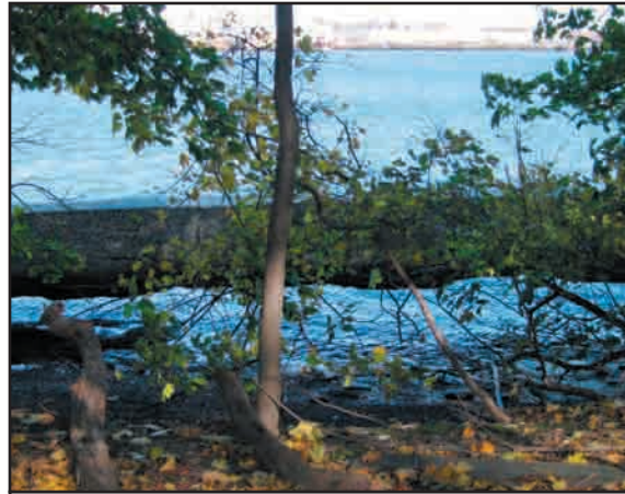
Figure 9: Breached seawall at north shore, view north (Christy Lombardo, 2005)
