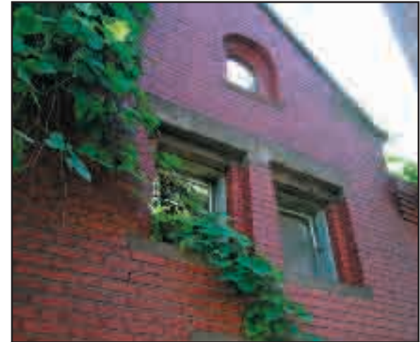
Kudzu and poison ivy overgrowth threatens buildings (Sarah Shotwell, 2005)
