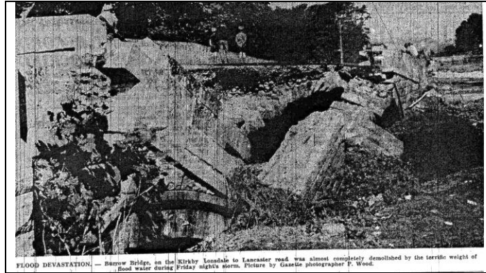
FLOOD DEVASTATION. — Birrow Bridge, on the Kirkby Lonsdale to Lancaster road, was almost completely demolished by the terrific weight of flood water during Friday night's storm. Picture by Gazette photographer F. Wood.
