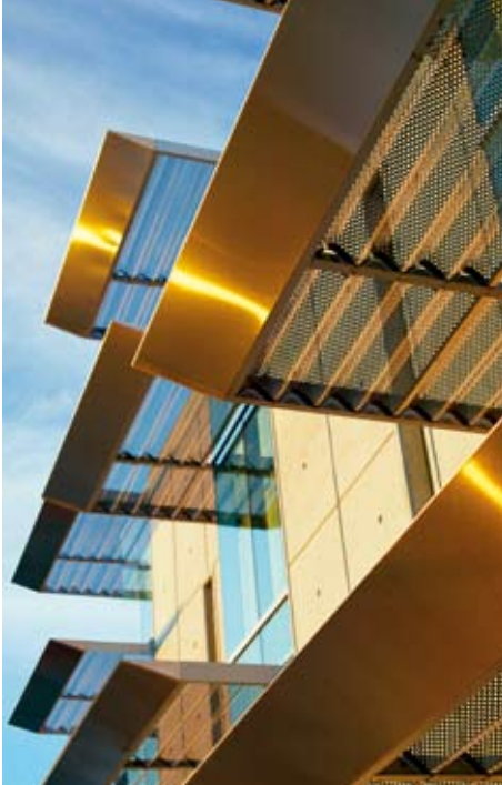
Corrugated and perforated steel sheets have been used for the horizontal sunscreens.
