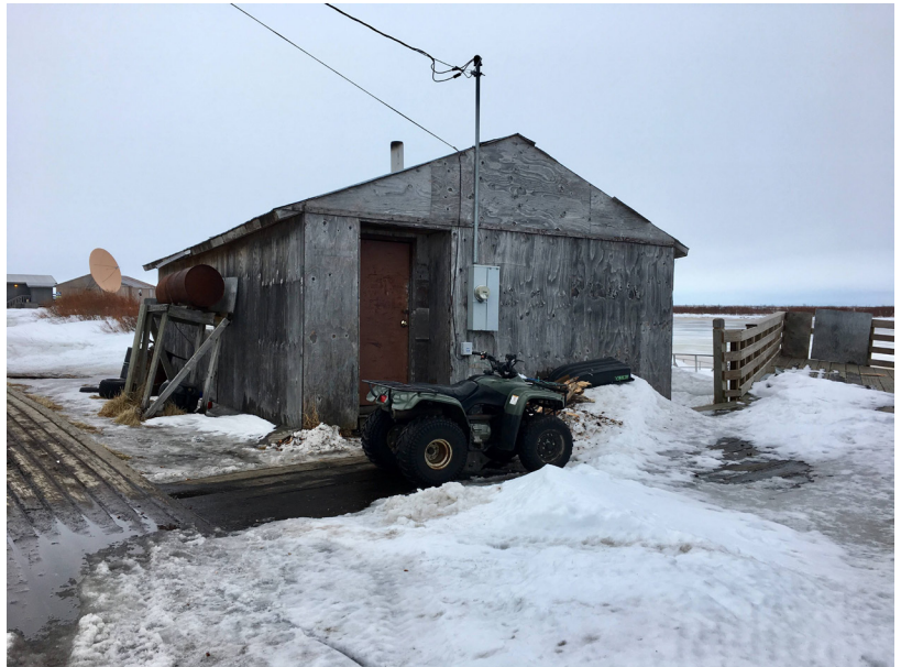
The Tribe's rental house has safety concerns that should be addressed immediately, including the need for a proper foundation, ventilation, roof repair, and a multi-wall flue for the wood stove.
