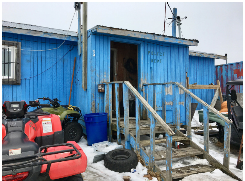
A retrofit of the police station could decrease its energy use by $883 per year .
