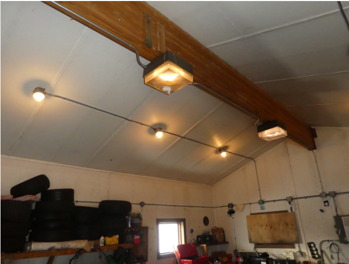
Ensure all lighting fixtures are working and replace any fixtures that are not.
