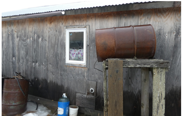
Visually inspect the house exterior and document any changes to the structure, such as current damage getting worse.
