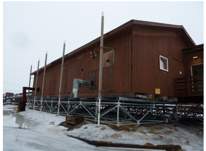
Visually inspect the building exterior and document any damage to the structure, such as damaged roofing or siding.
