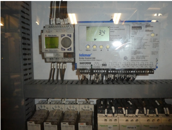
Ensure that the thermostat for the boiler is programmed to run at lower temperatures when there is no one in the building.
