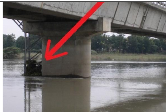
San Agustin bridge, Arayat, Pampanga with flood marks (debris) still clinging to the steel support of the WL sensor of Arayat telemetry station. WL peaked at 8.37 m. attained on 1600H of June 26th.
