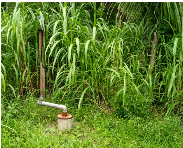
The Level III Basco Water System will soon provide sufficient and safe water upon the installation of the transmission and distribution lines.
