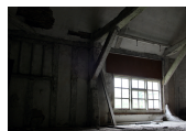
Interior shot of part of the upper storey in Grimston Hall, 2018. This is NOT accessible to the public.
