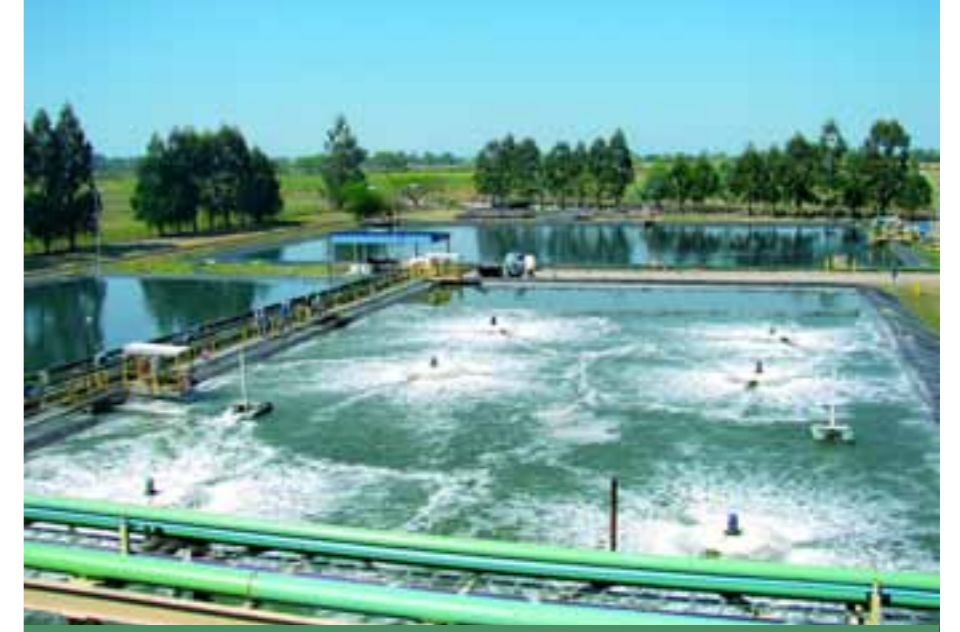
Filter plant located in Cruz del Norte, Province of Tucumán.
