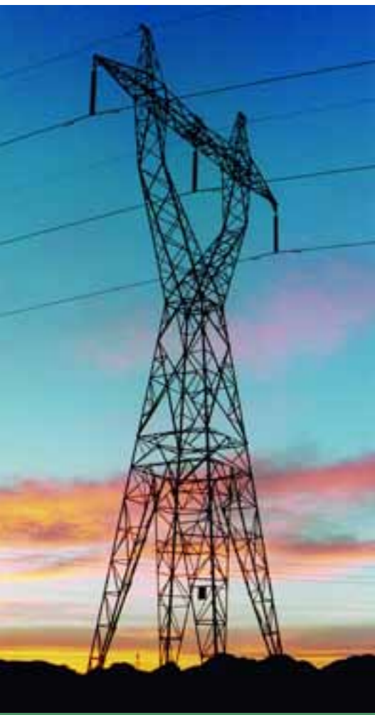
El Bracho-La Alumbra high voltage line is a 220 Kw line that covers 202 km from Tucumán to the mine.
