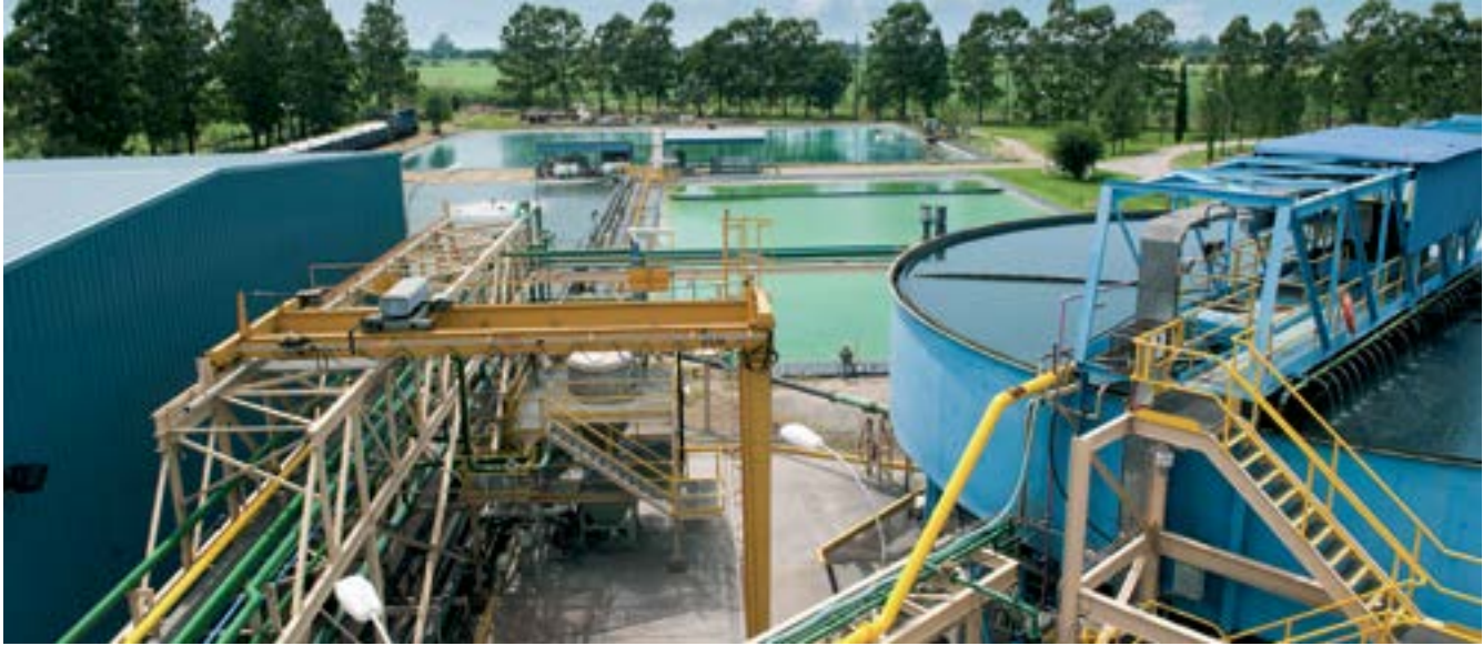
View of the Filter Plant, located in Tucumán, where the concentrate is dewatered and water is treated and subjected to quality controls at our ISO 17025 certified laboratory.
