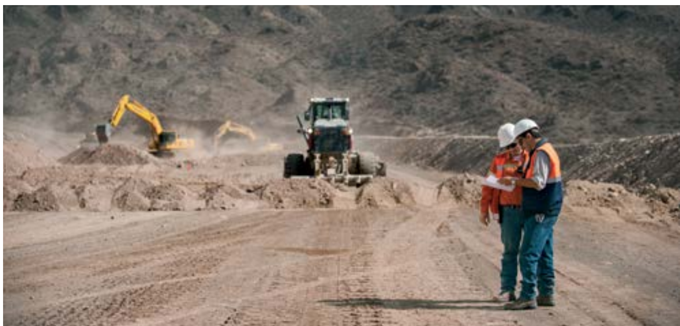
Daniel Andreola and Enzo Faedda overseeing the opening of roads to Bajo el Durazno.
