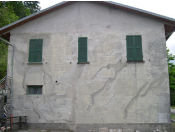
Figure 6 – Cracks in a house of Roccamurata.
