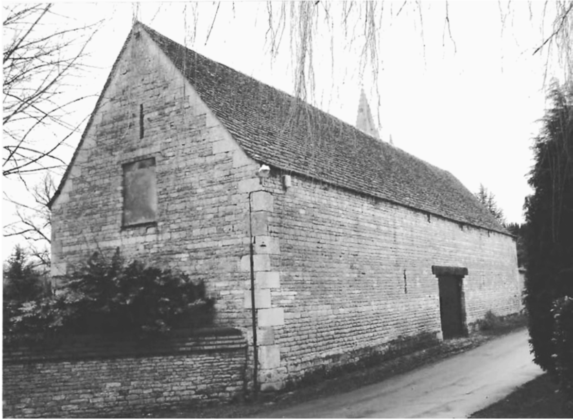
Fig. 7. Tithe barns such as this one at Empingham were necessary for the clergy when tithes were given in kind. By the early nineteenth century many tithes had been commuted to money payments, and some tithe barns, such as the one at Barrowden, were demolished (photograph: Robert Ovens)
