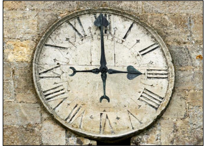
The engraved stone clock dial by Henry Stone on the south face of the church tower. (RO)
