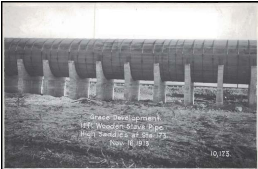
Figure 5.6 Utah Power and Light Company began expansion of Grace Plant in 1913. Note the concrete saddles supporting Flowline No. 2. (Courtesy PacifiCorp).
