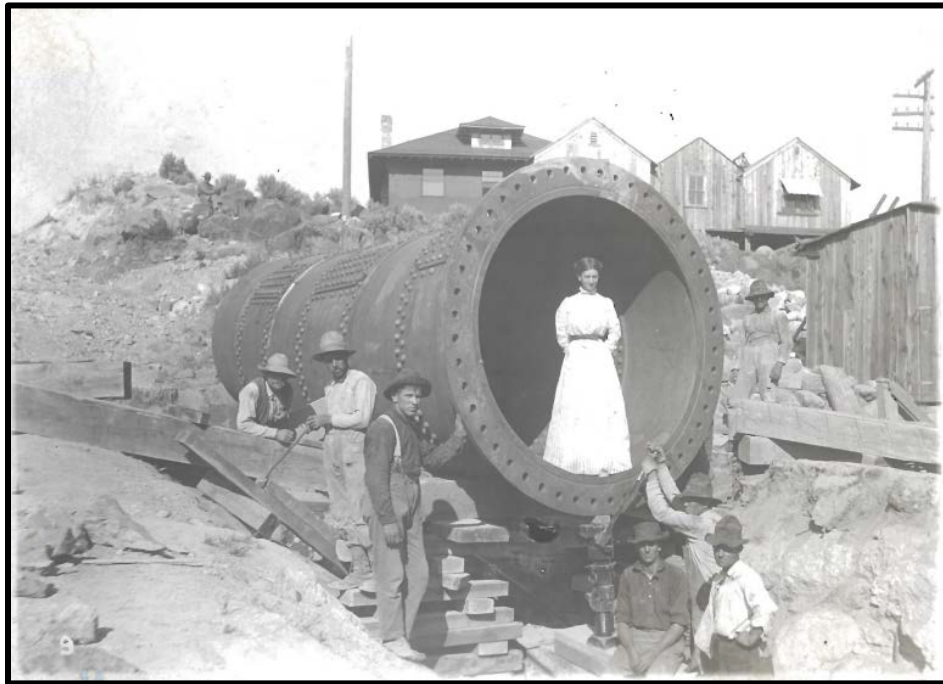
Figure 4.7 The immense size of the pipeline is shown in this photo taken during the 1907 construction. (Courtesy PacifiCorp).
