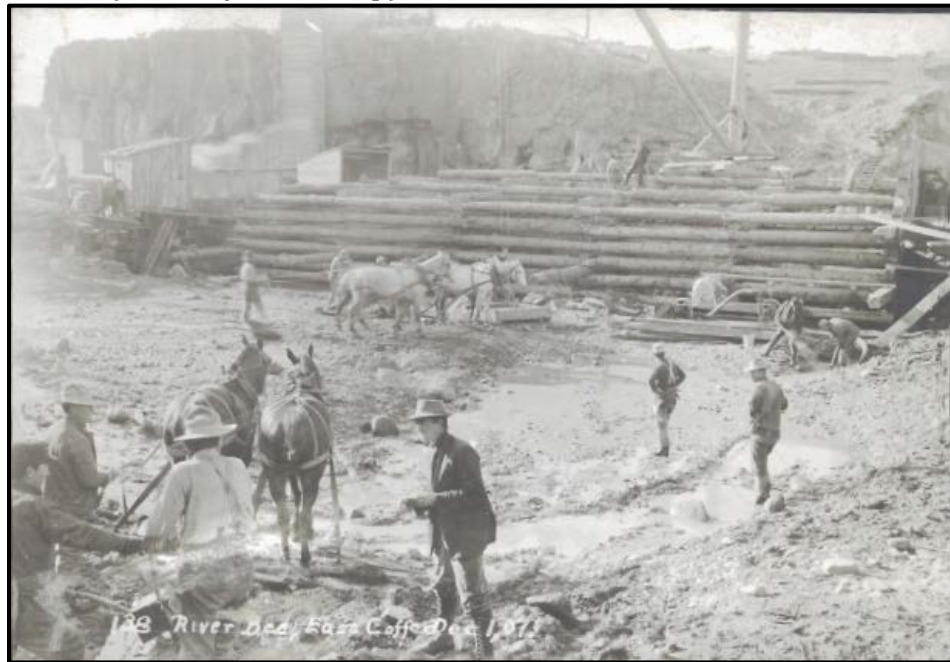
Figure 4.5 A cofferdam or coffer is a temporary structure constructed to facilitate projects in areas that are normally submerged. This 1907 photo shows construction crews standing in the riverbed near the east coffer. (Courtesy PacifiCorp).Chapter 4 Illustrations and Maps
