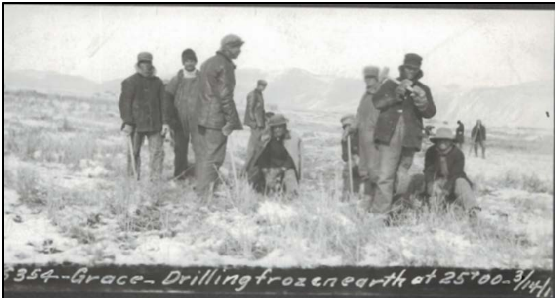
Figure 5.4 Men worked in all conditions during the construction of the expanded Grace Dam and Power Plant. (Courtesy PacifiCorp).
