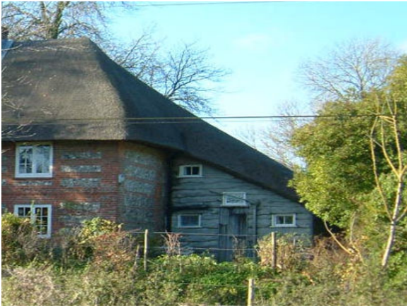
Flint Cottage. Although this type of timber clad lean-to is not unusual for such thatched cottages the waney-edged weather board and the slot shaped windows are not traditional in the area and not particularly appropriate to the listed building.
