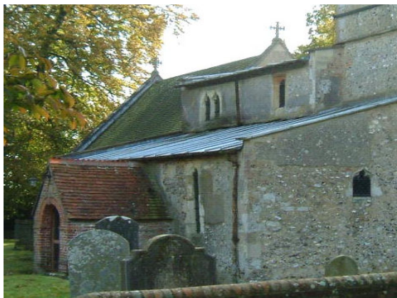
A roof of cast lead with welted seams. Walls are of flint, chalk and greensand stone rubble rendered in lime with limestone dressings
