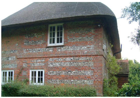
Thatch over a flint and brick banded wall. Timber casement windows with glazing bars
