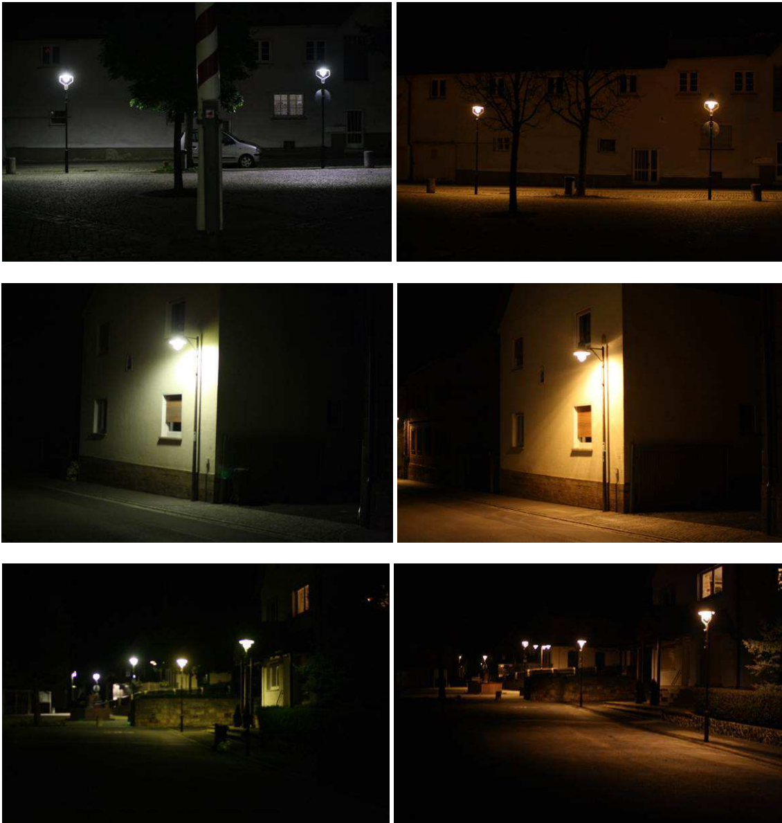
Fig. 9.7: Old HQL lighting in Oberelsbach (left side) has been replaced by 3000 K LED (right side). In the top left picture, in the right side a luminaire with a test LED kit with 4000 K was installed. The pictures on the right were taken using double exposure time (1/10 s) compared to the pictures on the left (1/20 s)
