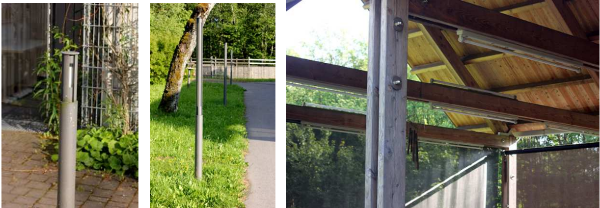
Fig. 9.1: Outdoor lighting at the environmental education center, which has been removed.
