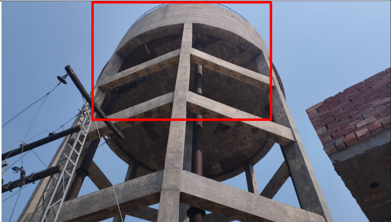
Figure 9 [Missing Water Gauge at Reservoir]
