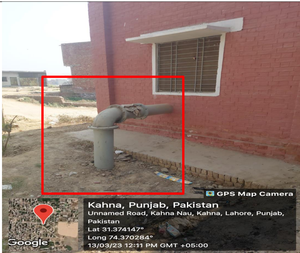
Figure 6 [No Valve Chamber was observed]
