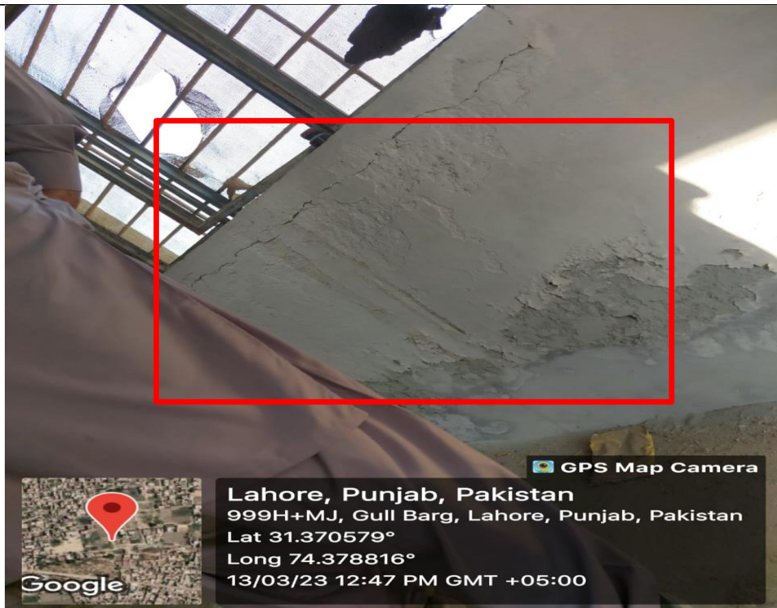
Figure 02 [Efflorescence and Spalling of the Plastering work]
