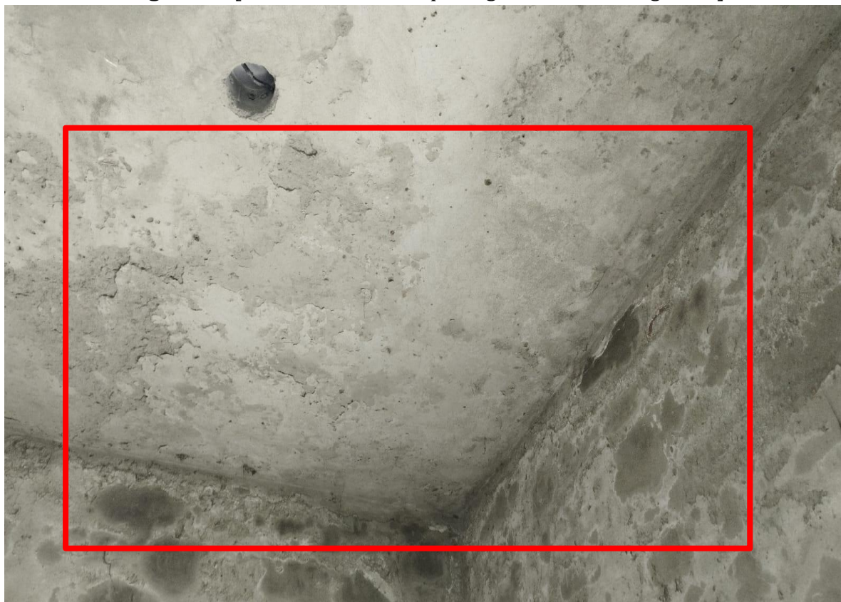
Figure 03 [Efflorescence and Spalling of the Plastering work]
