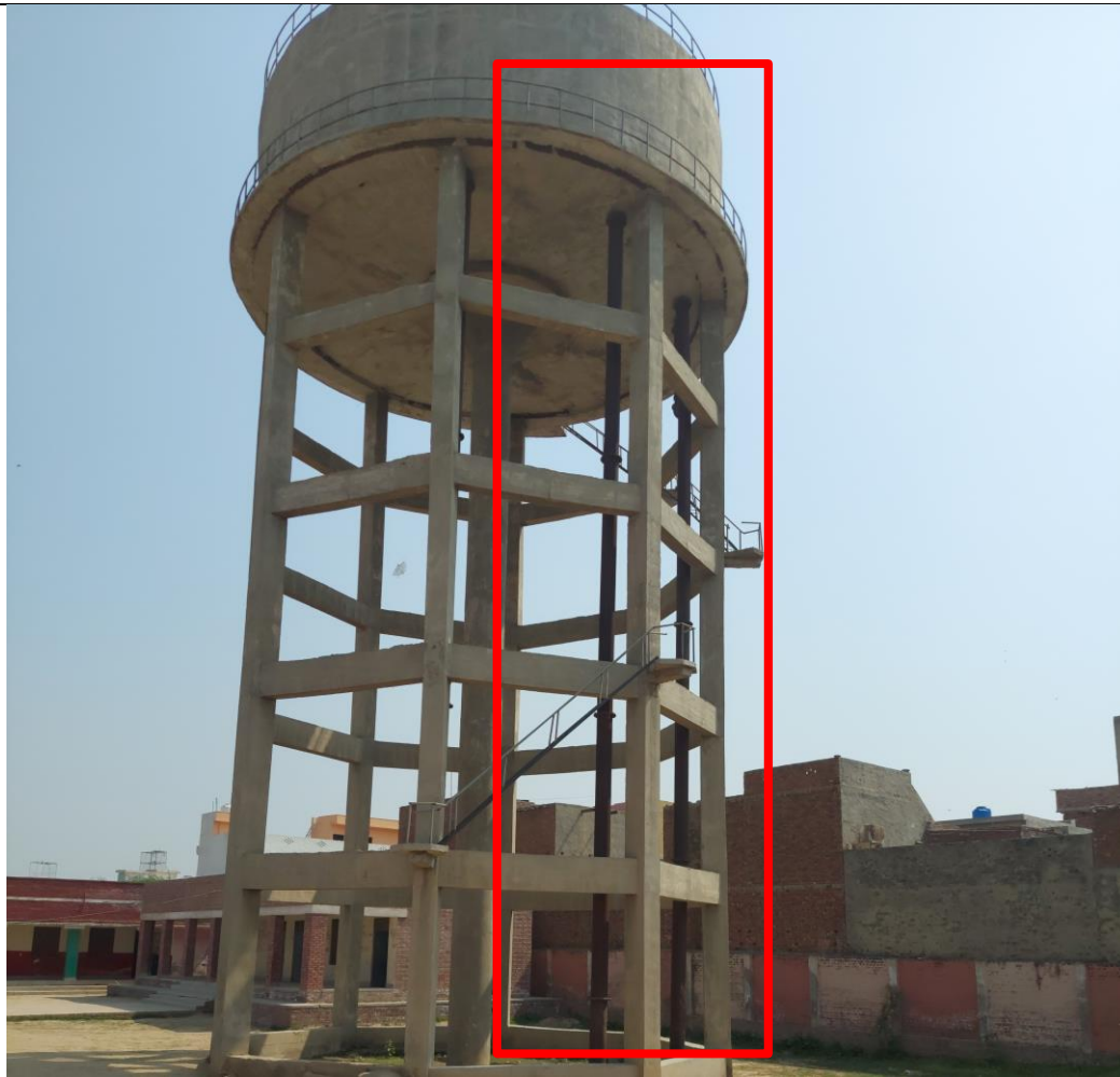
Figure 8 [Missing Anti Rust Paint on the Steel Rising Main]
