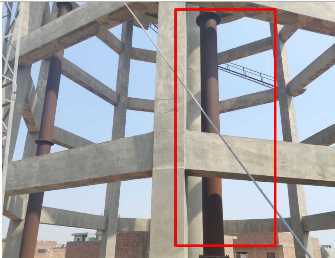
Figure 7 [Missing Anti Rust Paint on the Steel Rising Main]
