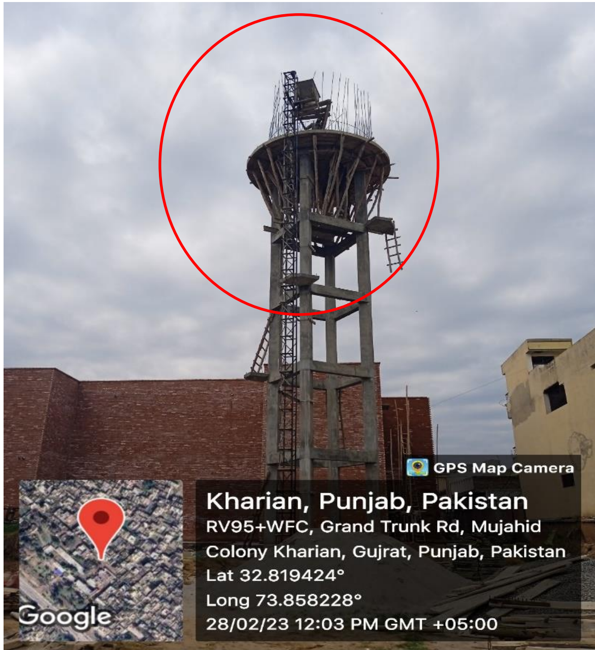
Figure 10: Laborers were working at height without PPEs
