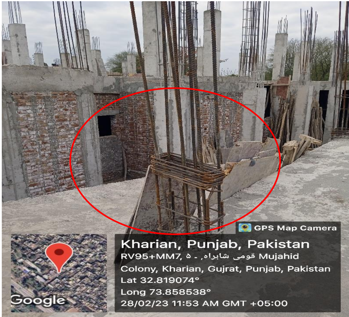
Figure 4: Incorrect Location of Vertical Lap in Column
