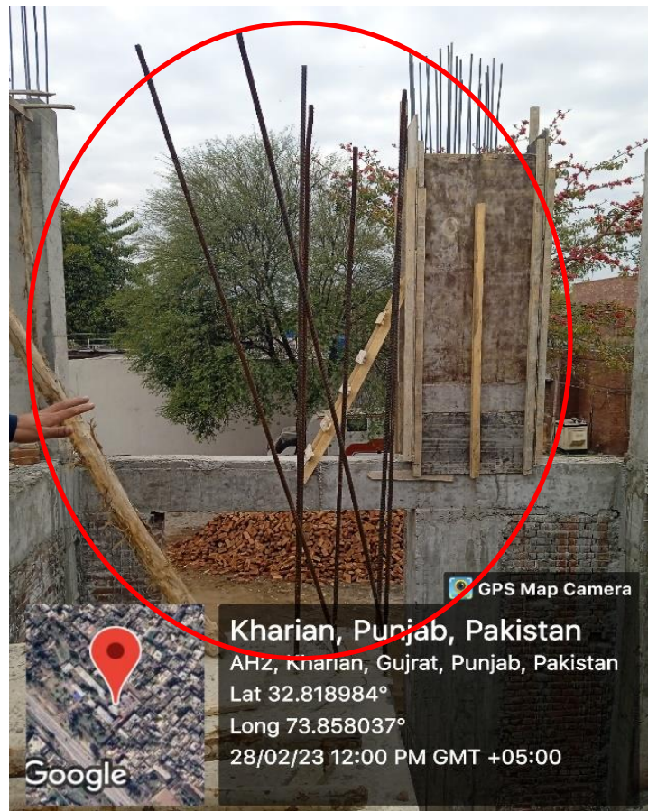
Figure 7: Dislocation of reinforcement of column cage due to non provision of cover separators
