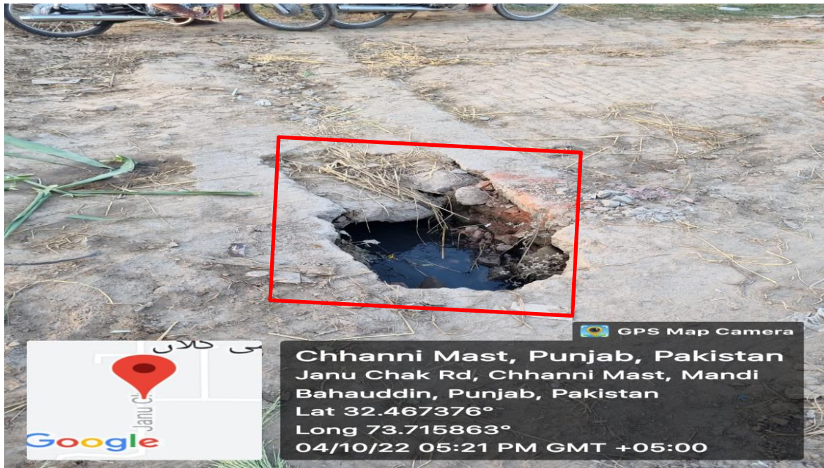
Figure 5: Broken Culvert of the Drainage
