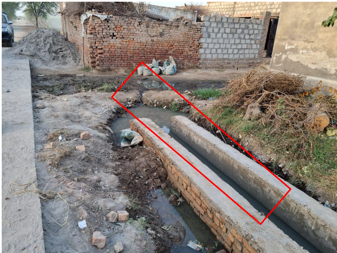
Figure 6: Drainage at Road and Houses Side (No Exit Point)
