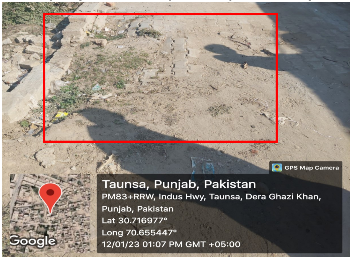
Figure 5 [Damaged and Settled Tuff Tiles in Streets]
