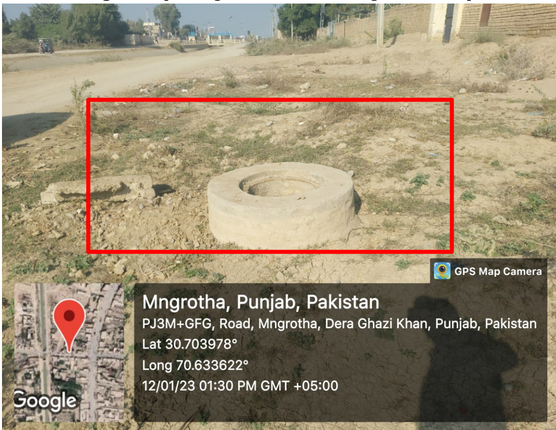
Figure 03 [Missing Manhole along with the Canal Road]
