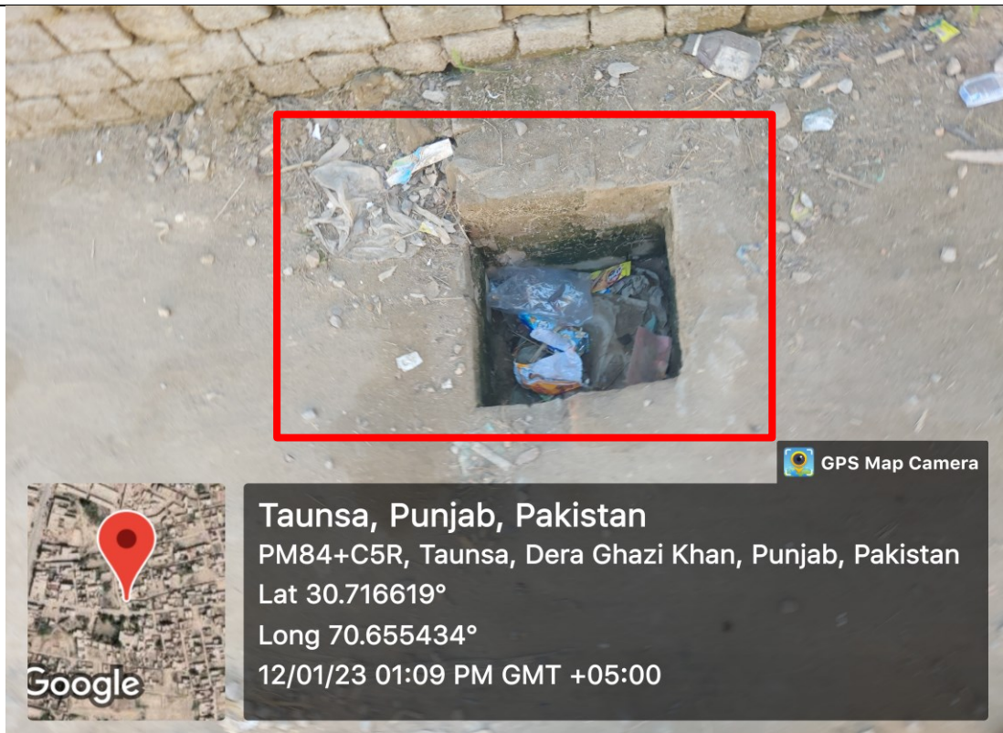
Figure 7 [Grating was missing on Gully Grating Chambers ]
