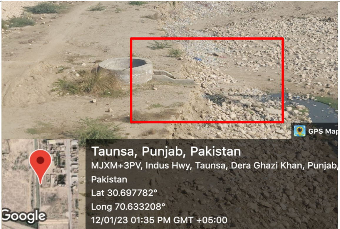
Figure 9 [Damaged Sullage Carrier]
