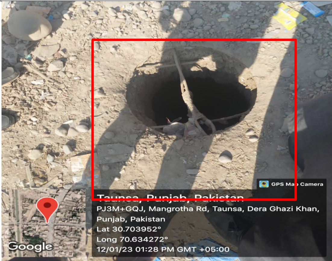
Figure 02 [Missing Manhole Cover at Magrotha Chowk]
