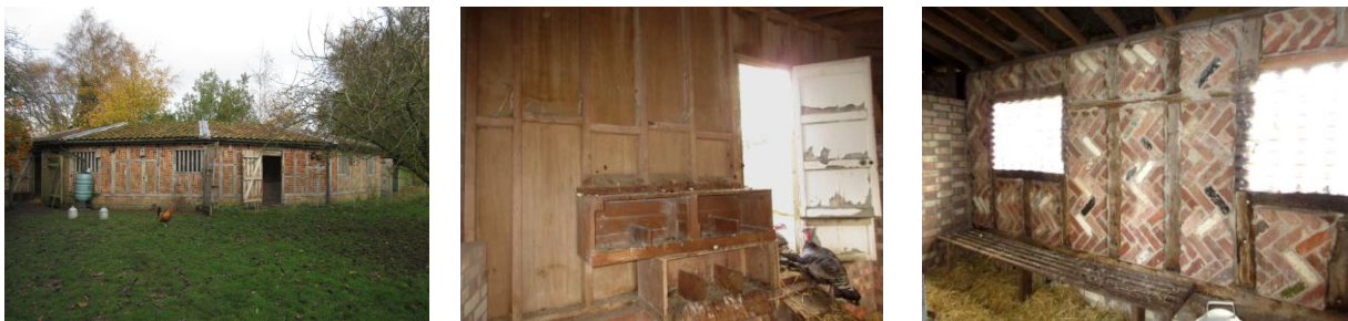
Left: elevations 4, 5 & 6; Centre: NW wall of compartment 6; Right: SE wall of compartment 6
