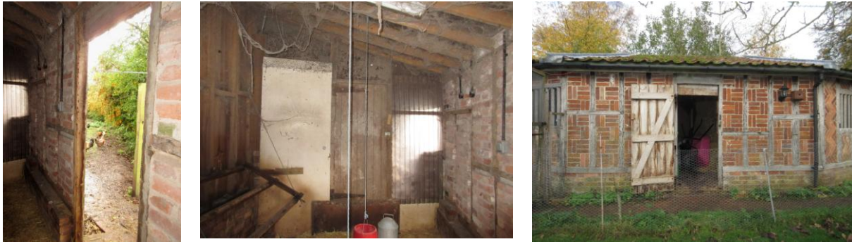
Compartment 3: Left: doorway showing single skin brick exterior wall; Centre: interior looking SE; Right: external SW elevation
