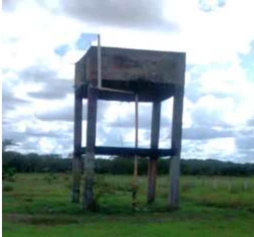
Photograph 36: Water storage tank, Aceitico Police Precinct
