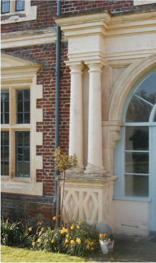
Fig. 15. The Clock House, detail of stonework showing Blomfield's inserted arch moulding, corbel and set back jamb standing back from the mouldings of the plinth to the paired side columns. Richard Garnier .
