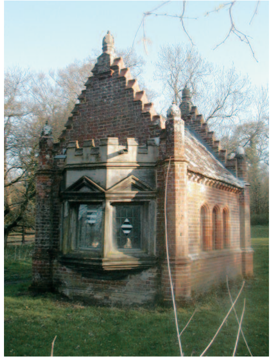
Fig. 21. Shell House from north-west, with oriel window of wood conforming to that added by Blore to the porch of the house. Richard Garnier.
