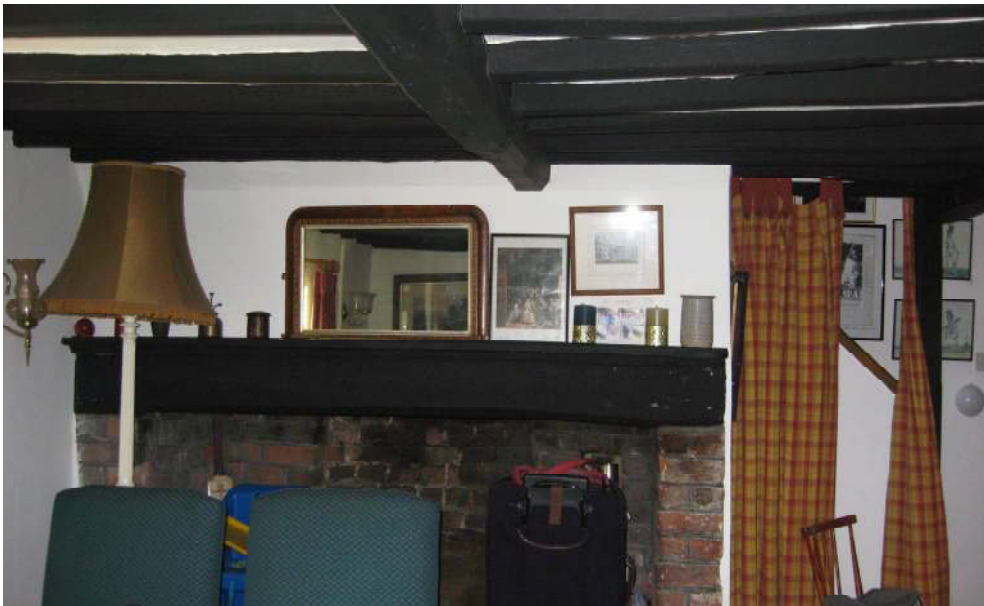
The above photograph is of the large inglenook fire place at the former gable end of the one-bay ground floor room. Beyond the opening is the modern staircase, which rises between the stack and a itchen extension of uncertain date.
