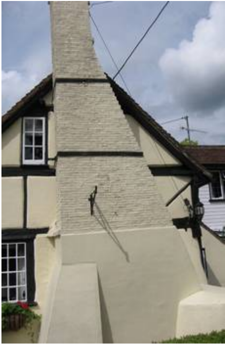
East gable with stack and queen strut truss 7 (mostly hidden by the stack, but intact inside)
