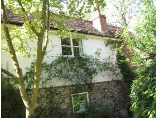
Rear, east elevation. B.& F wall of outshut with raised brick wall and new roof above and modern inserted g.f. window
