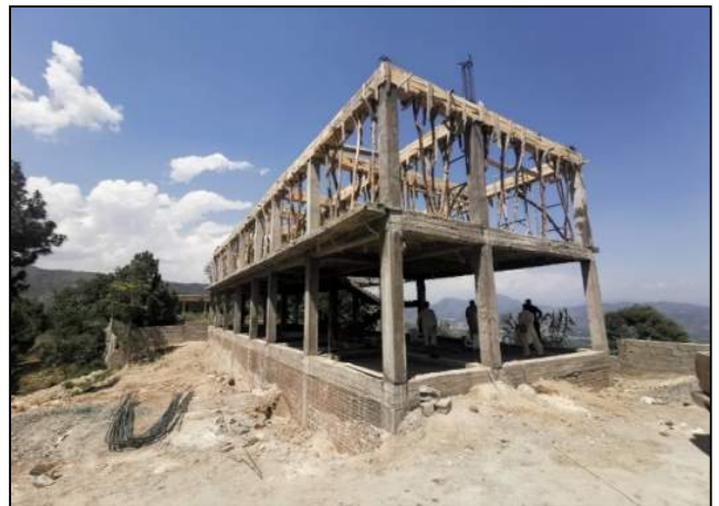
Fig. 48. View of the Module T-3 at GPS Pir Patay Qalagai, Swat
