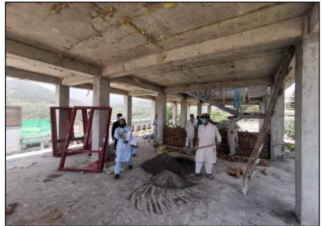
Fig. 46. Brick work in progress at SF of module M-13 at GGPS Shah Dherai, Swat
