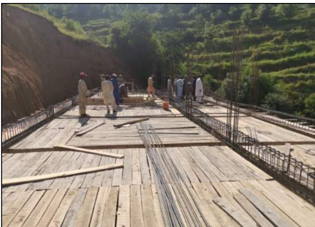
Fig. 53. Formwork and rebar work for GF slab in progress for T3 at GPS Fatima, Swat
