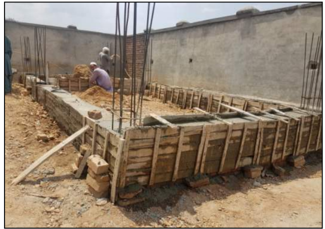
Fig. 28. Concrete surface exhibiting poor workmanship -GGPS Maroba, Nowshera
