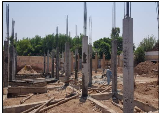
Fig. 30. Honeycombing at M-3 (H) columns-GHS Masho Khel, Peshawar
