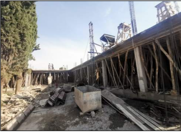
Fig. 55. Rebar work for F/F columns in progress for U-Shaped Building GGCMHS, Thana Malakand
