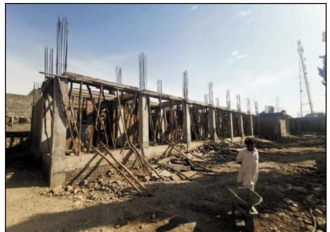
Fig. 54. Formwork for G/F Beams in progress for M6 (H) GGCMHS THANA, MALAKAND
