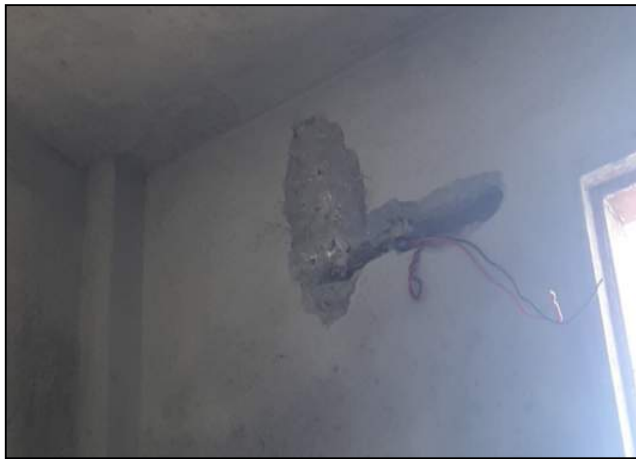
Fig. 09. Plastered surface being damaged for locating light points - GPS Yari Koroona, Peshawar
