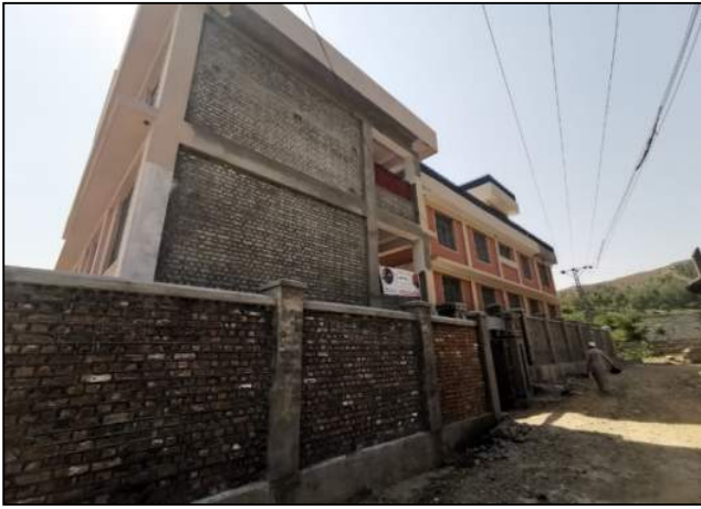
Fig. 43. Works in progress at Module M13 B. View of GGPS Bara Bandai, Swat
