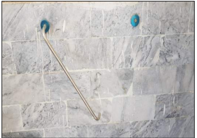
Fig. 40. Towel rod is broken-GPS Jhoke Umaray Wali, DIK
