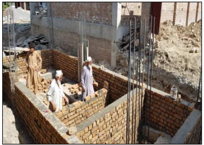
Fig. 18. Brick work and concreting of short columns in progress-GHS Khesghi Bala, Nowshera
