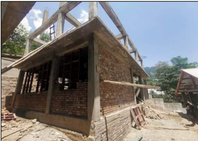
Fig. 51. Brick masonry works along with fixing of door and window frames in progress at G/F of T-7 for GPS Chatoria, Swat
