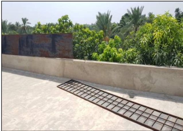
Fig. 39. Steel grill on parapet wall is broken-GPS Jhoke Umaray Wali, DIK
