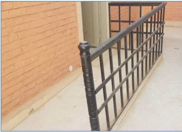
Fig. 37. Steel railing for ramp is not stable-GPS No.01 Yarak, DIK
