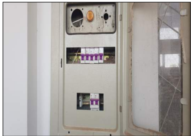
Fig. 36. Change over and voltmeter were found missing - GPS No.01 Yarak, DIK
