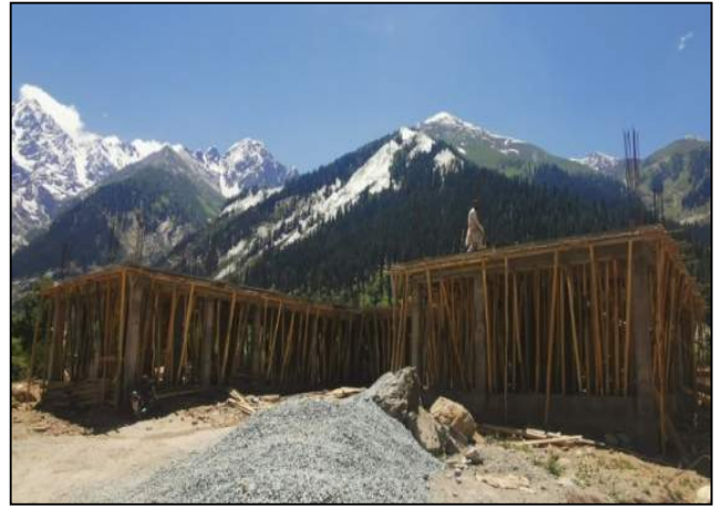
Fig. 56. G/F slab concrete works completed for U-Shaped Building at GHS Matiltan, Swat
