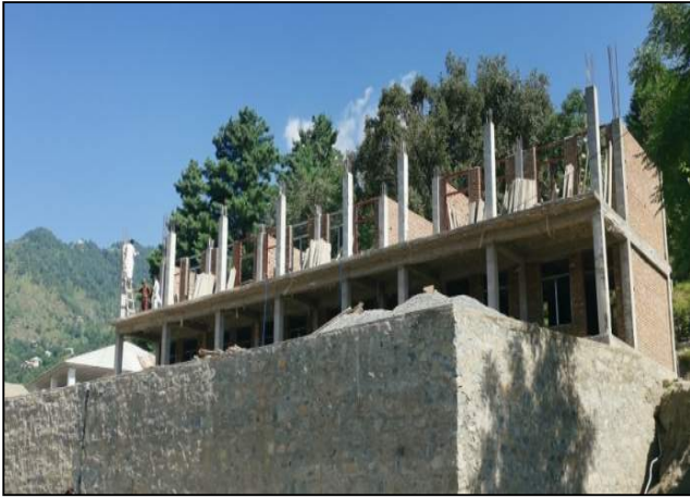
Fig. 49. Formwork for truss beam in progress – view of the Module T3 at GPS Pansat, Swat
