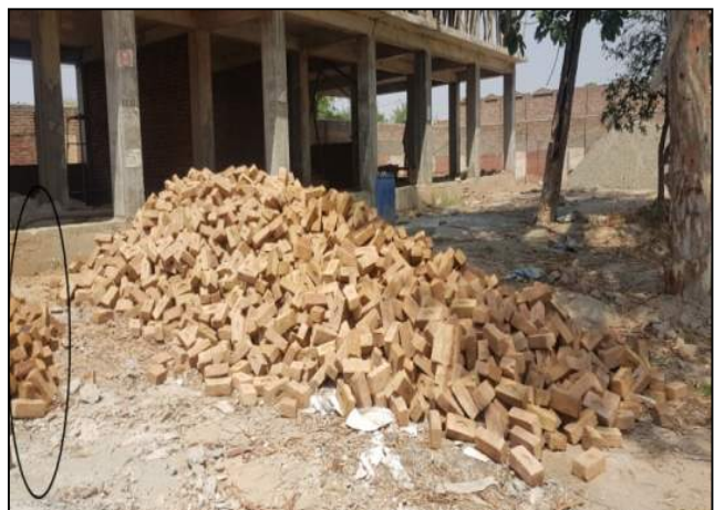
Fig. 34. Rejected brick encircled-GHS Matani, Peshawar
