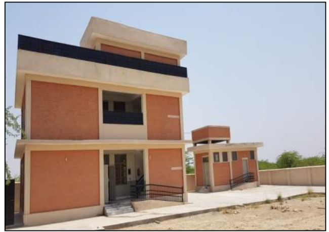
Fig. 38. Steel railings should be strengthened-GPS Bairoon Sharqi, DIK
