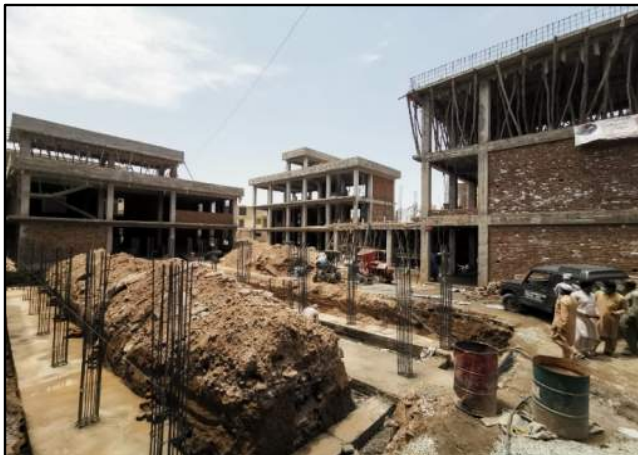
Fig. 41. View of Modules M-6, M-11, M 13 A, B and C at GGHS No. 1 Mingora, Swat
