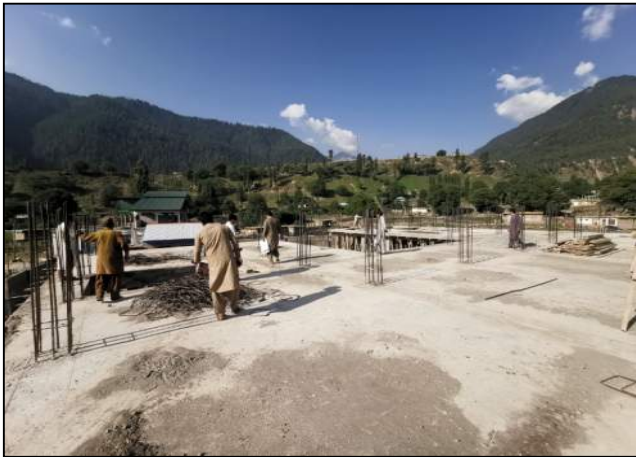
Fig. 57. Commenced rebar work for F/F columns of U-Shaped Building at GHS Utror, Swat
