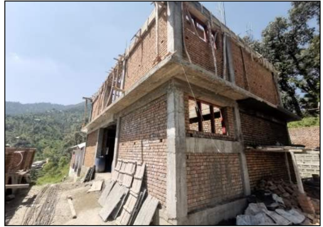
Fig. 50. T7 roof truss beam formwork along with the external plastering works in progress at GPS Talkar, Swat
