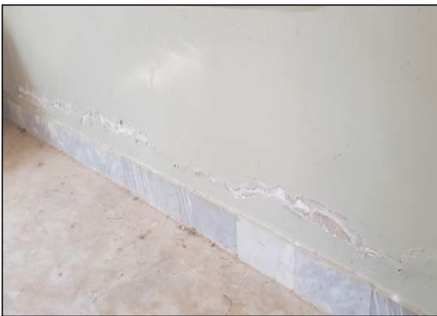
Fig. 35. Painted surface deteriorated above the skirting level-GPS No.01 Yarak, DIK
