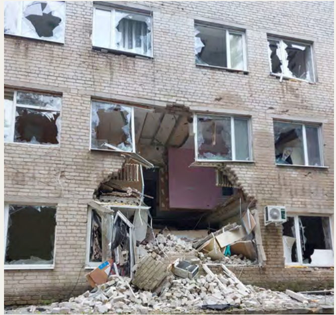
Severe destruction of one of the buildings of the Balakliia Clinical Multiprofile Intensive Care Hospital, which was allegedly hit by a tank. Photo captured by the hospital's medical personnel in September 2022.
