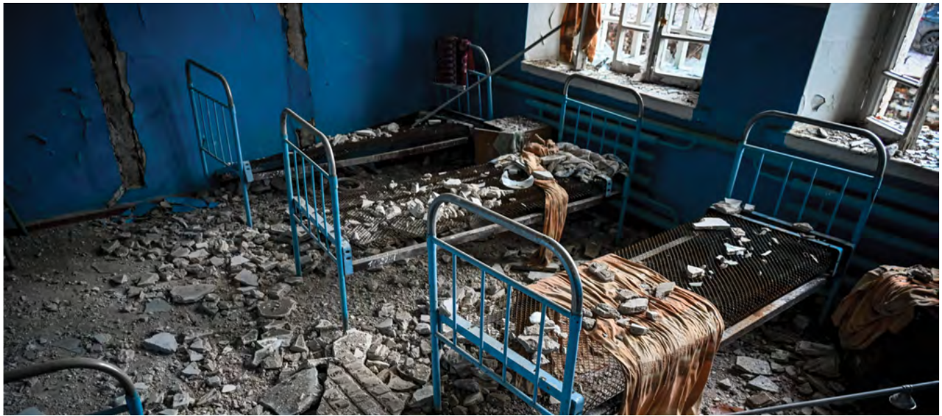
A room in a damaged hospital building near Kupiansk, in Kharkivska oblast. Photo captured on December 15, 2022 by Sergey Bobok/AFP/Getty Images.
