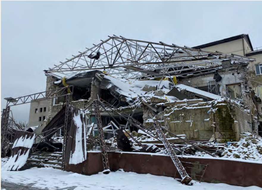
Top: Destroyed exterior of the Izium Central City Hospital, which was damaged in at least three attacks in March 2022.
