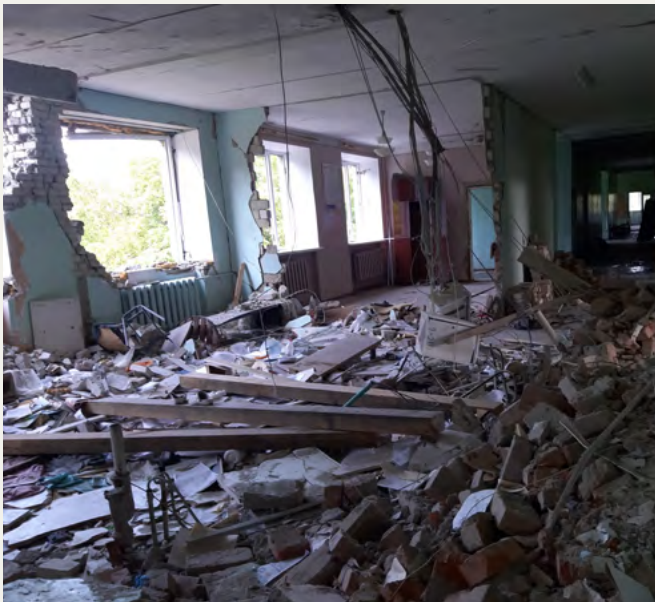
Top: Damage to the exterior of the Trostianets City Hospital. Photo captured by the Ukrainian Healthcare Center in August 2022.
