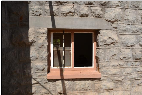
Figure 28. Small window with wide and over-designed cement lintel (Photograph: M. Naude 2013)
