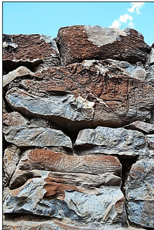
Figure 22. Interior of the wall exposing dolomite stone used for the construction of the annex to the dwelling (photograph: M. Naude 2013)
