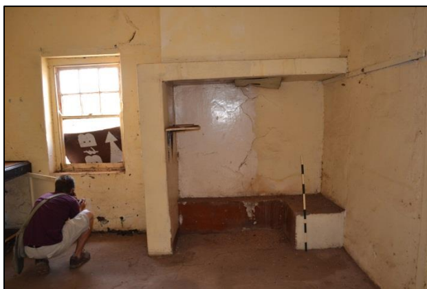
Figure 38. Alcove of the first hearth - in the kitchen - which was later altered to accommodate a coal stove (Photograph: M. Naude 2013)
