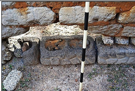
Figure 19. At the base of the structure some of the prefabricated cement bricks used for the additions to the dwelling are exposed where they have been used as foundation material for this structure (Photograph: M. Naude 2013)
