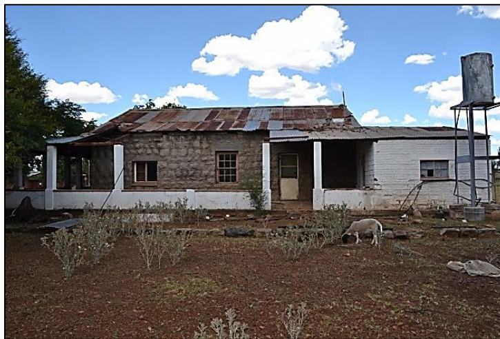
Figure 12. Back elevation of the dwelling indicating the location of the core dwelling (grey dolomite stone) and bath room stoepkamer (white-washed room)
