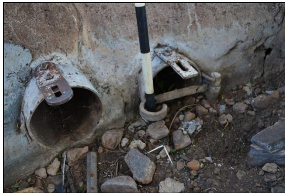
Figure 15. Pipes letting water from the principal water furrow into secondary furrows (photograph: M. Naude 2013)
