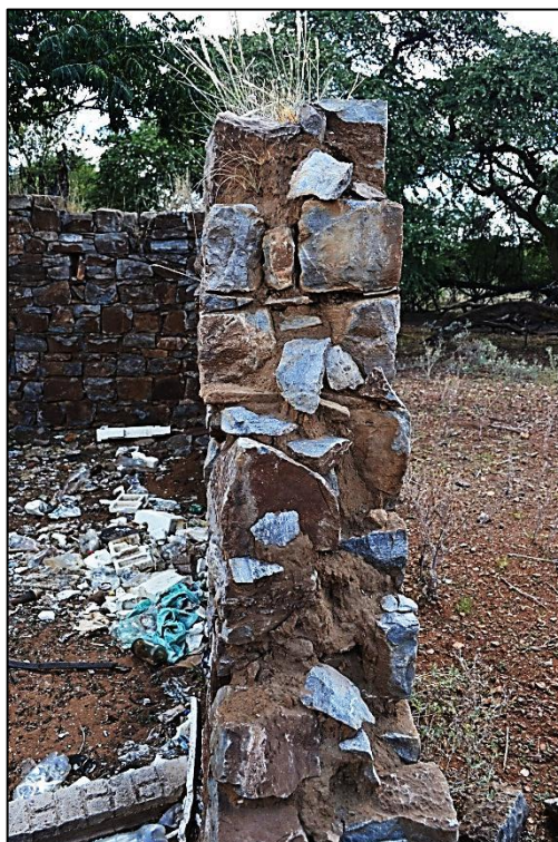
Figure 23. Section through the dolomite wall construction of the annex indicating the use of clay mortar with the stone (photograph: M. Naude 2013)
