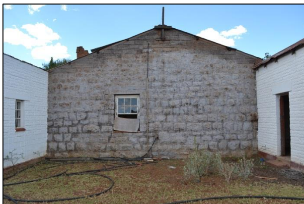
Figure 43. Side gable of the original dwelling and the two stoepkamers added to the back and sides of the core section of the dwelling (photograph: M. Naude 2013)
