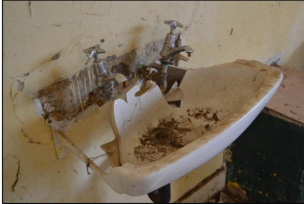
Figure 35. Vandalized porcelain wash basin in the bath room (Photograph: M. Naude 2013)
