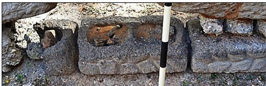
Figure 20. Detail of prefabricated cement bricks used for the foundation of the structure (photograph: M. Naude 2013).
