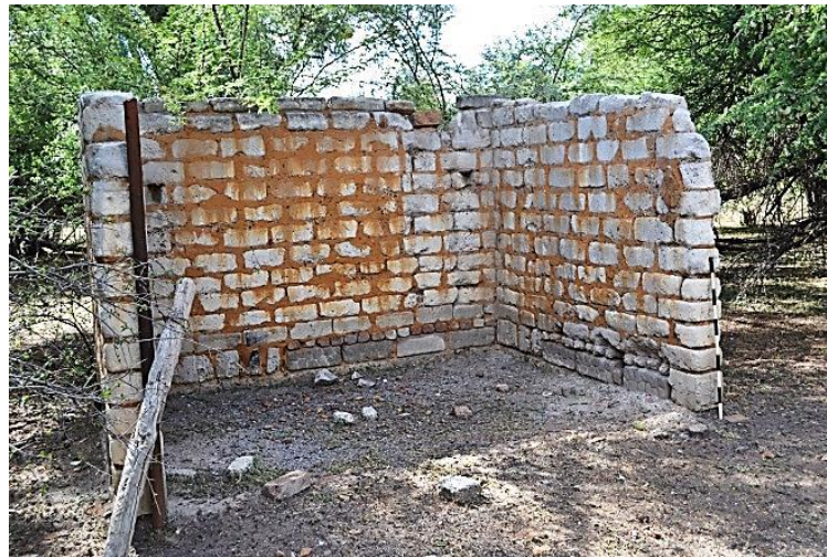
Figure 6. Ruin of what seems to be an unfinished or vandalized outbuilding constructed with clay bricks
