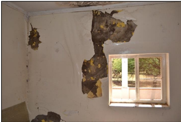
Figure 36. Large areas of the walls of the later additions have been penetrated by rain water due to bad drainage, guttering and roof problems (Photograph: M. Naude 2013).
