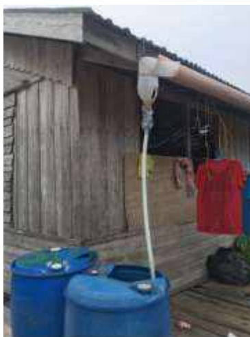
Rudimentary rainwater harvesting system for household use like laundry and cleaning.
