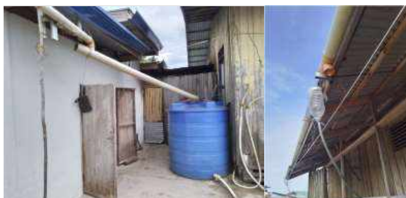
Figure 4.7. Examples of rudimentary rainwater harvesting systems in Sibutu and Sitangkai
