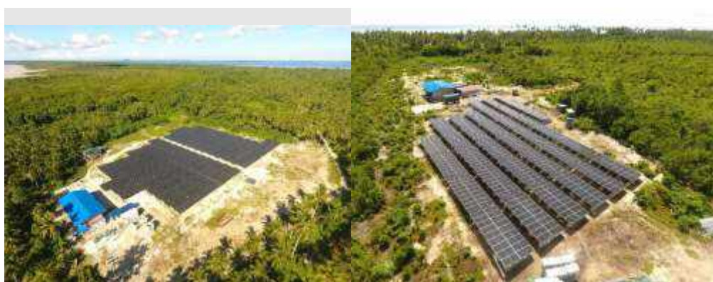
Figure 14. Photovoltaic plants and diesel generators deployed by the RETS project in Sibutu and Sitangkai, as of October 2021. Source: The RETS project
