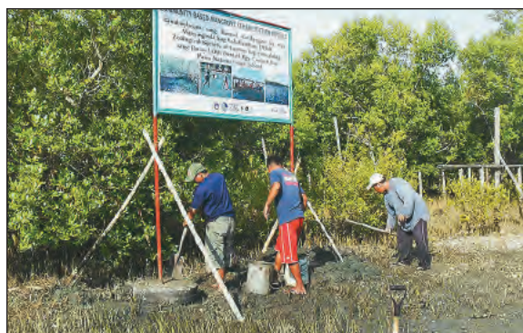
FIG. 58. PO members of Buntod Katibyugan and staff of LGU Panay install billboard of the mangrove project in Buntod, Panay, Capiz, 16 April 2011.
