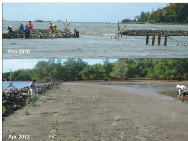
FIG. 33. Two lengths of breakwater, 0.9 m high by 1-2 m wide by 70 m and 110 m long, have consolidated sediment and provided both substrate and protection to planted and natural mangrove recruits in Pedada, Ajuy, Iloilo.
