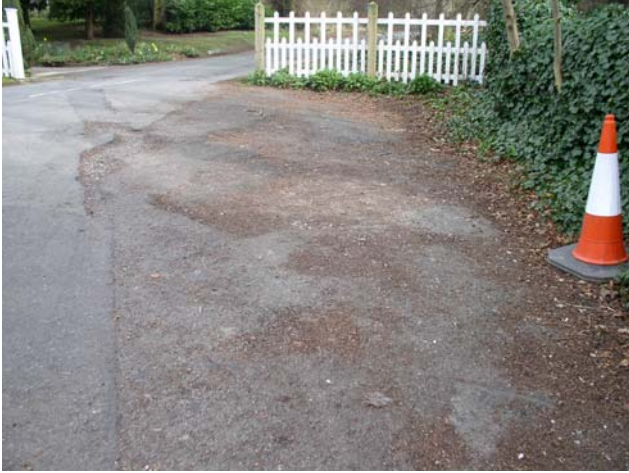
Vale Royal Drive entrance – requires re-surfacing
