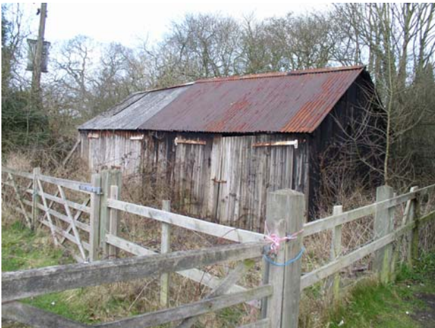
Untidy shed to the rear of the Mews
