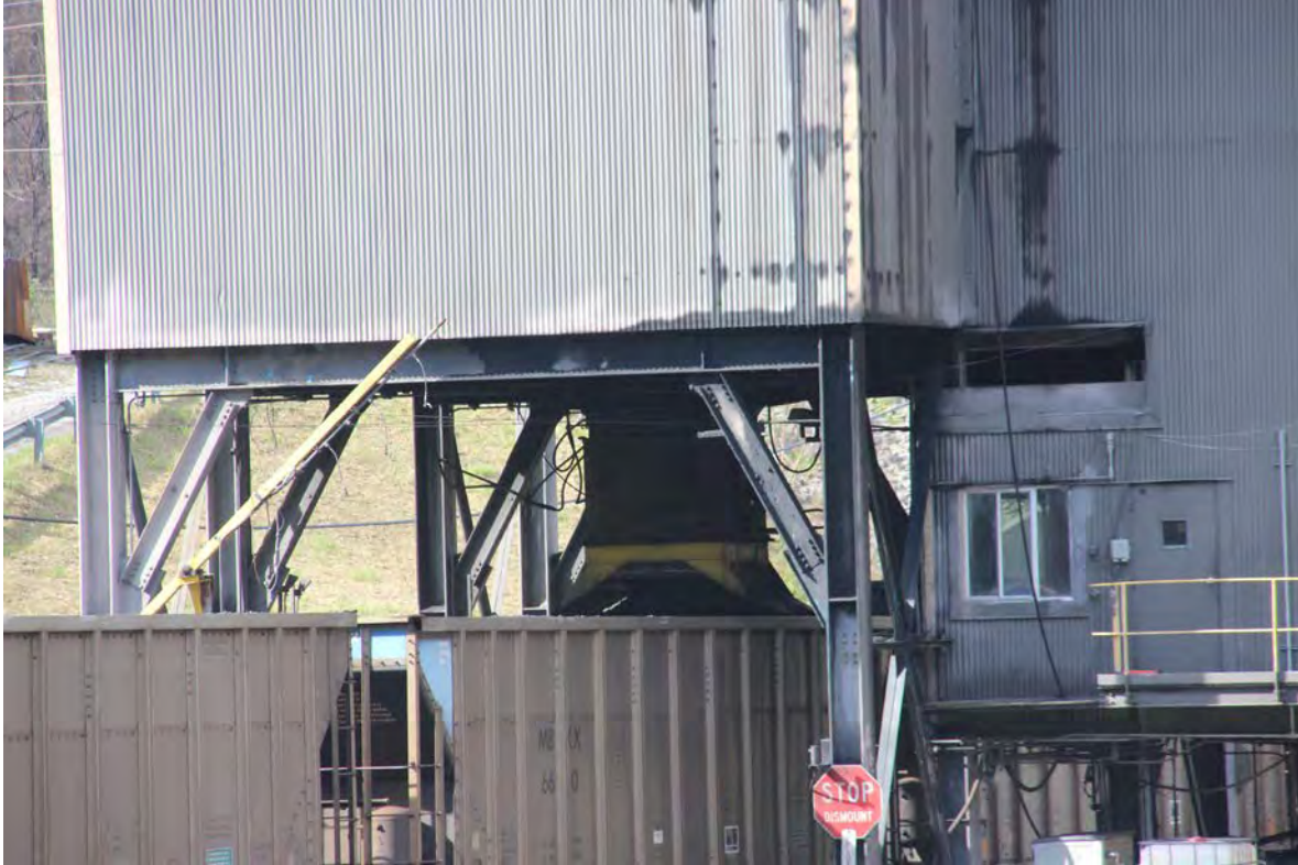
Another view of the flood loader at work. The coal is carried from the storage area to the flood loader by conveyor belts. The whole operation is controlled by a computer that ensures the right amount and type of coal is loaded into the hoppers.
