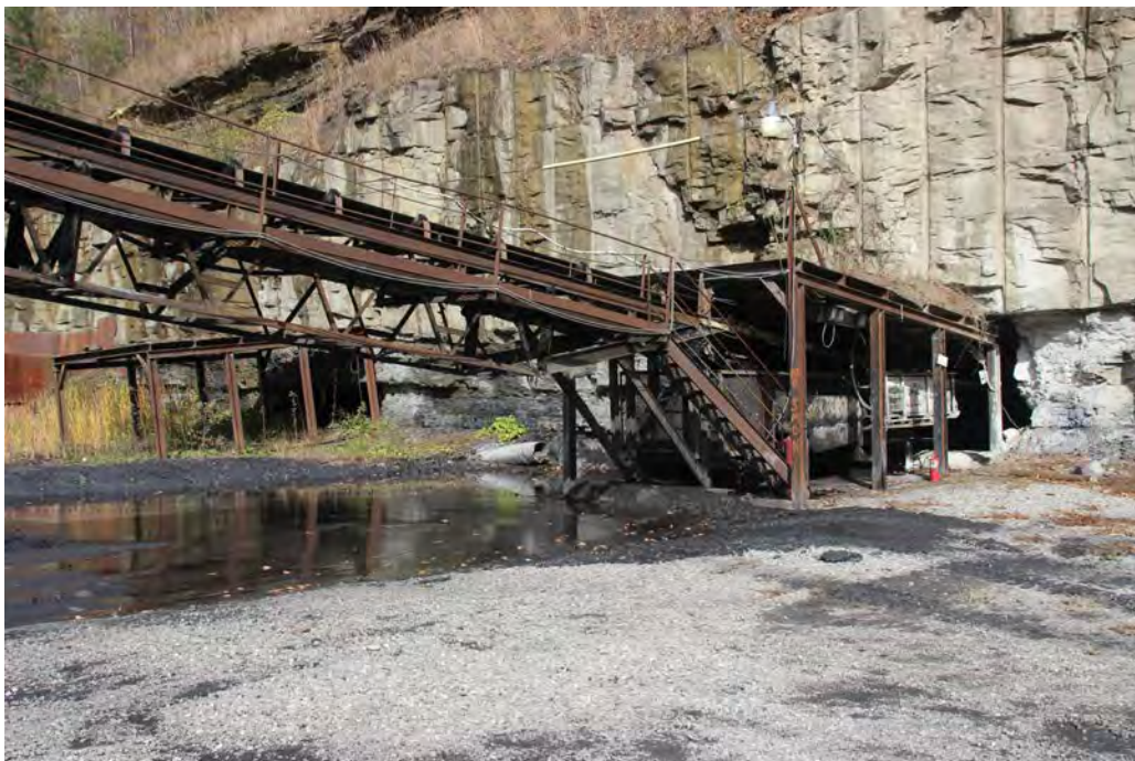
The conveyor belt that carries the coal mined from inside the mine to the wash plant. The open iron skeleton shed in the background was the previous site from which the conveyer belt exited the mine.
