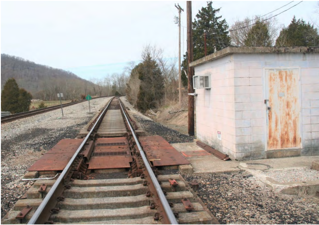
A view down the track toward Ravenna. The weight scale house on the right.
