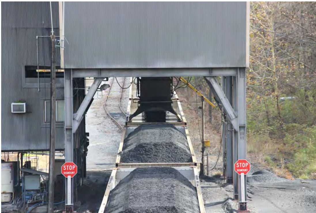
A close-up of the flood loader. The hopper is pulled through the flood loader at 2 MPH. A computer fills the hopper with the right amount of coal, forming a smooth layer of coal at the eve of the hoppers.
