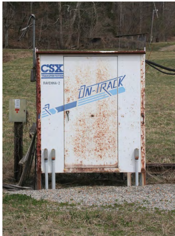
The signal box that controls the weight in motion scale
