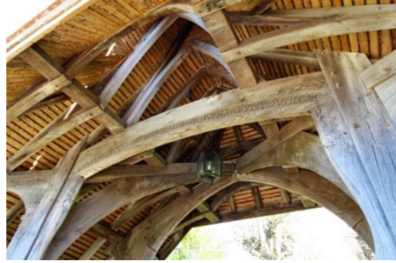
Roof structure of the Lych Gate to Saint Mary and Saint Peter's Church
