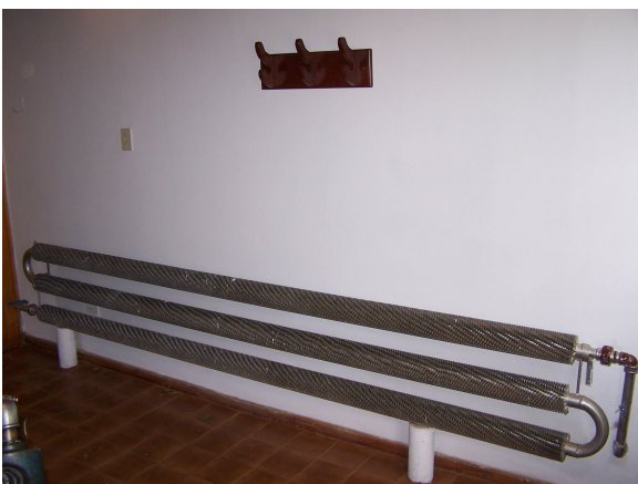
Figure 4: Heater of a hut of Aguas Calientes.
