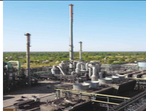
DCDA Gas Conditioning Plant (GCP) with 100 mt Stack Height
