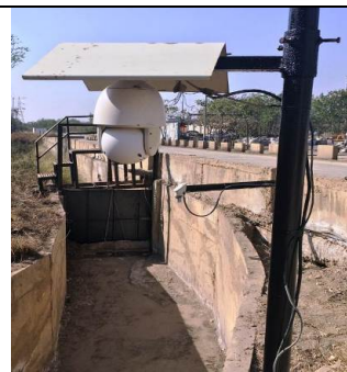
Flow meter Camera & installed at Plant O/1
