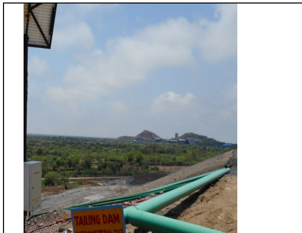
Taling dam pipeline
