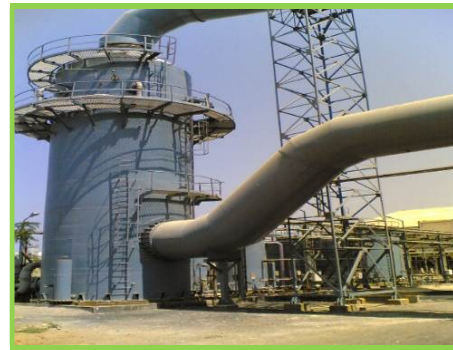
TGT Plant Scrubber
