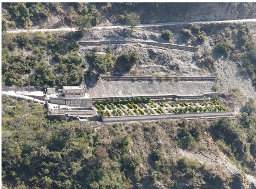
1.4 MLD Soil Based Technology STP
