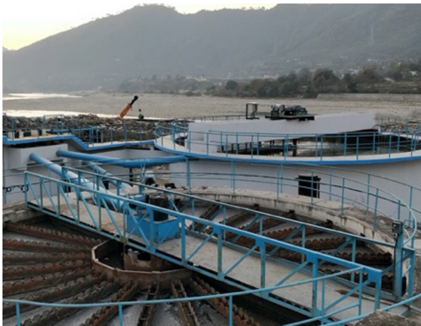
MLD STP Plant in Srinagar
