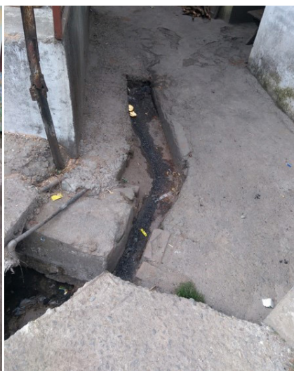
HHs discharging grey water into open drains
