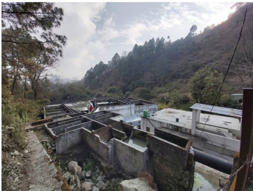
Sewage Treatment Plant (1.25 MLD), Bhimtal
