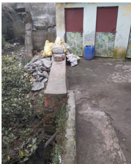
: HHs discharging grey water into open drains
