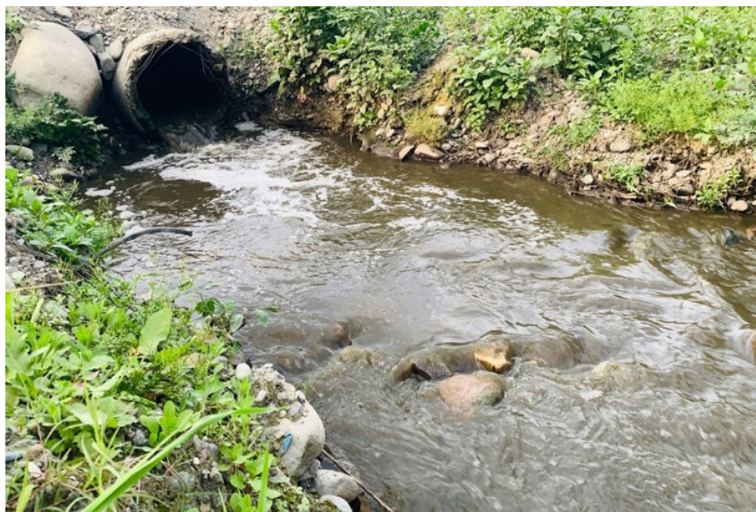
Image 7: Wastewater flowing into Gaula river through sewer lines
