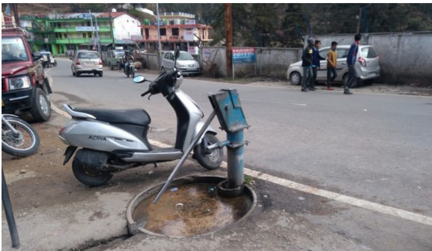
Public Hand Pumps installed by Jal Sansthan
