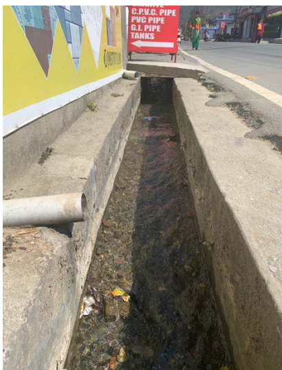
Open drains for grey water
