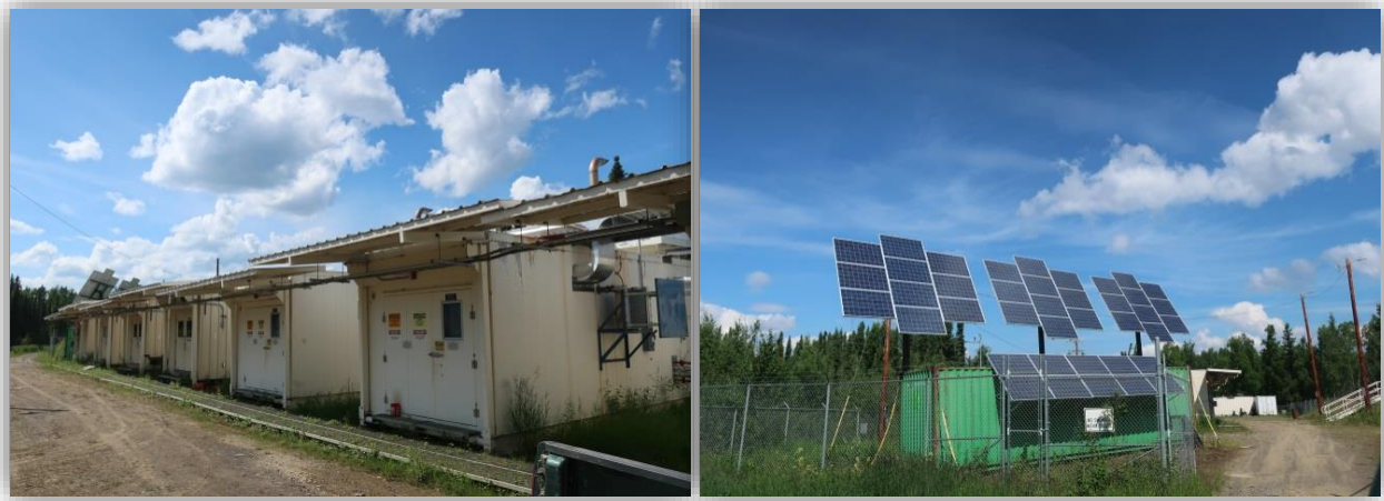
FIGURE 15 KALTAG POWER PLANT
