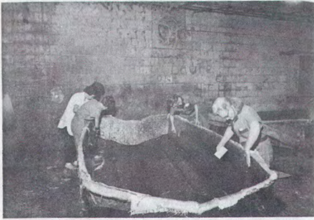
After inside of mold is sprayed with paint, a fiberglass mat is sprayed over paint and then, as shown here, a layer of woven roving is added, followed by a coating of clear resin, for impact strength.
