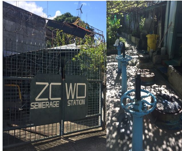
Figure 19: Sewage Pumping Station
