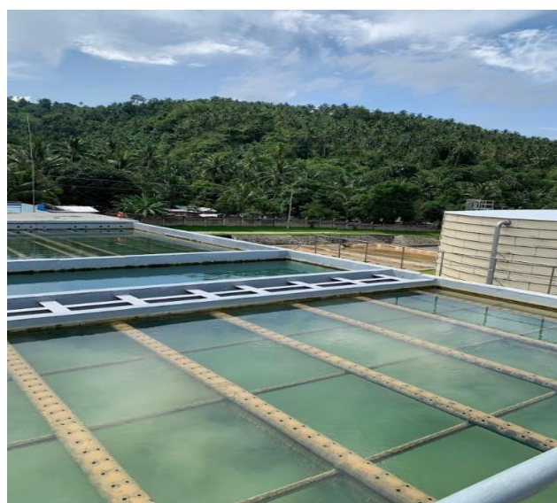
Figure 28: Prime Water 50 MLD Pamucutan Bulk Water Facility
